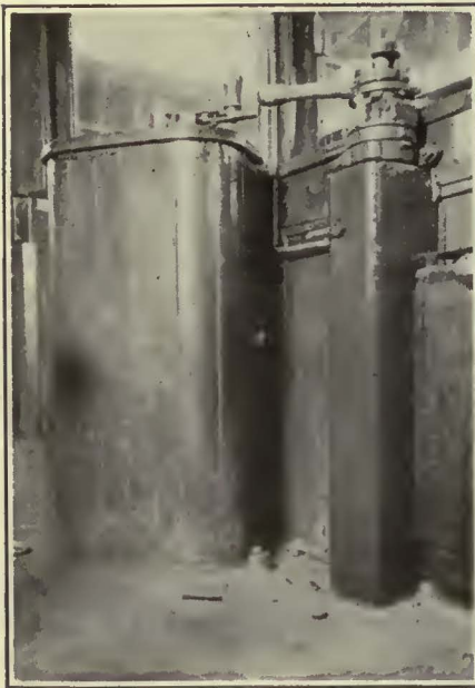
A Sheet-Iron Casing Over the Piping for Air Brake Valves and Inclosure for the Space Behind the Controllers Improve Platform Appearance of Cars in Detroit
