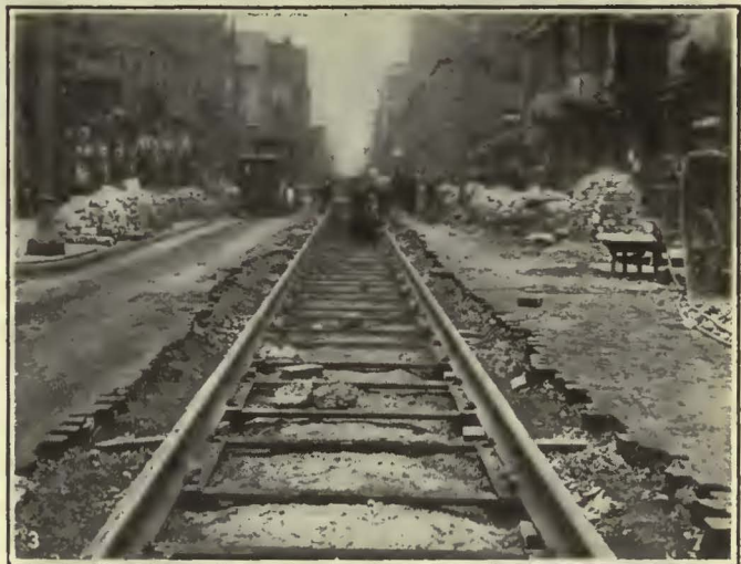
Various Stages in the Rebuilding of the Track on North Eleventh Street, Philadelphia
