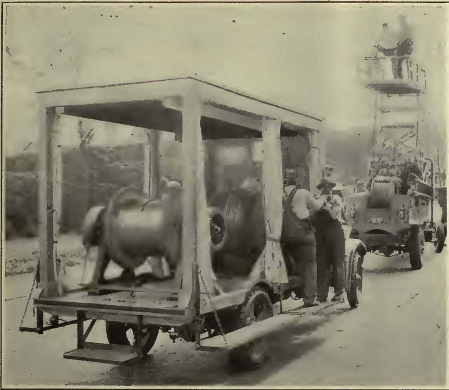
New Trolley Wire Stringing Truck Just Placed In Service by the Cleveland Railway
