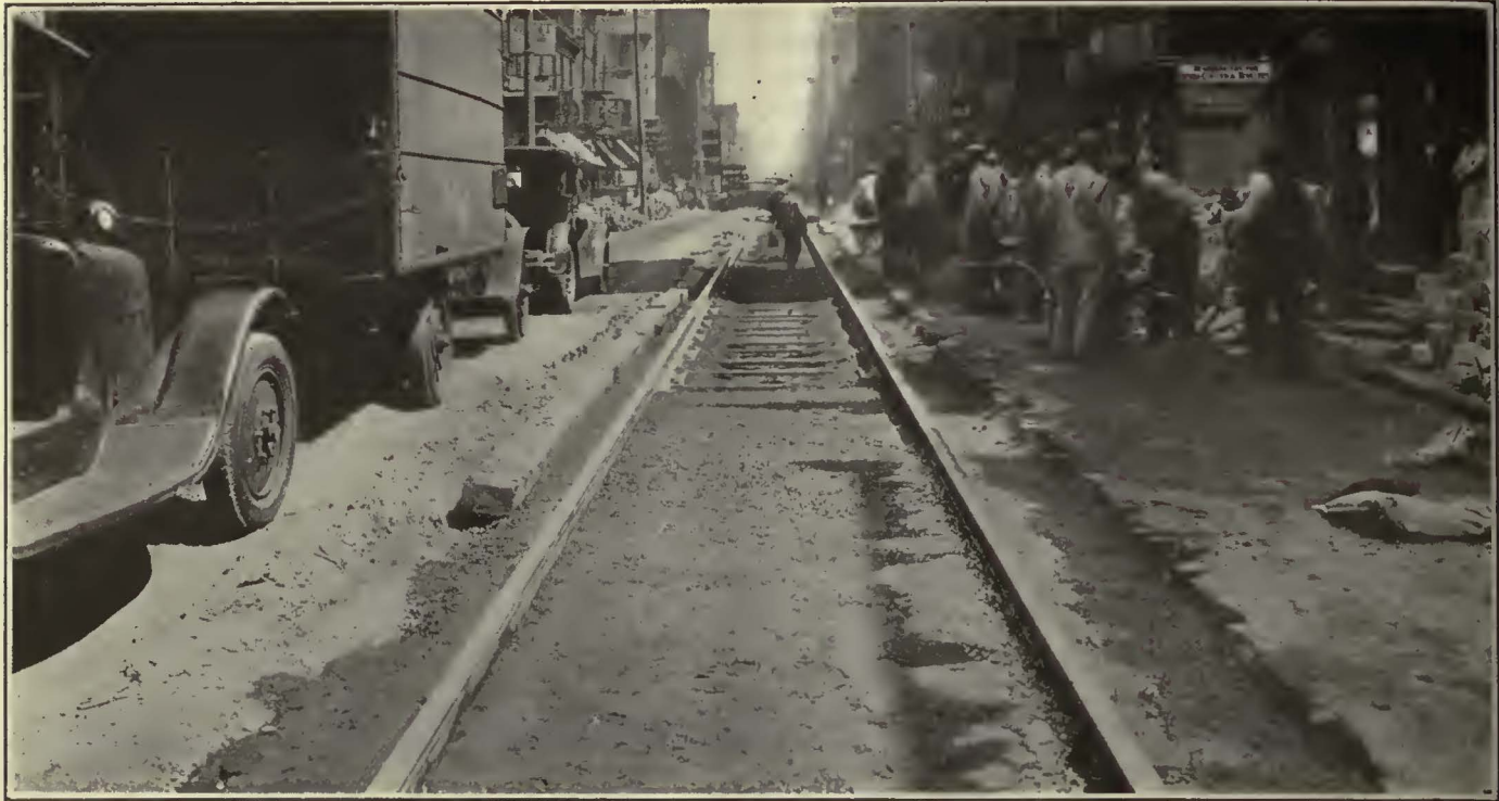
In the Foreground the Paving Base of Concrete Has Been Poured. Ahead of This Work Is the Twin Steel Tie Construction Thoroughly Tamped with a Dry Mix of Lumnite Cement and Traprock screenings
