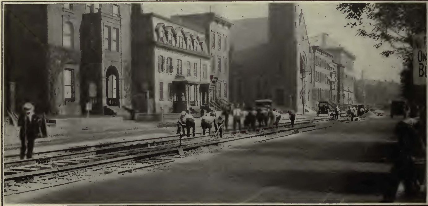
Tamping Ballast Under the Ties of the New Track on North Washington Street
