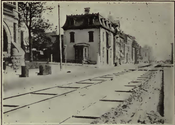
A Curb Separates Railway Area that Is Paved with Granite Block from the Rest of the Street Paved with Asphalt. This Shows the New Track on South Washington Street
