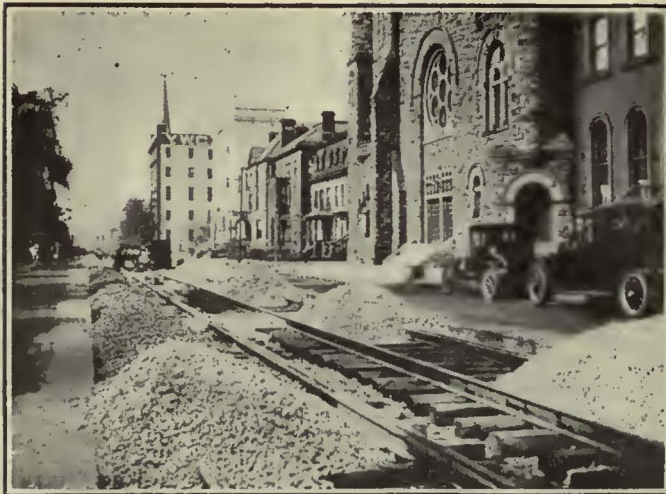
Track Structure Consists of 7-In. 101-Lb. Tram Rail on Wood Ties with Stone Ballast. This Is the Present Standard Type of Construction of the Railway for Use in Paved Streets
