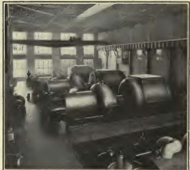
Four 10,000-Kw. Turbo-Generators Are Installed in the Narrows Plant and Space Is Provided for a Fifth
