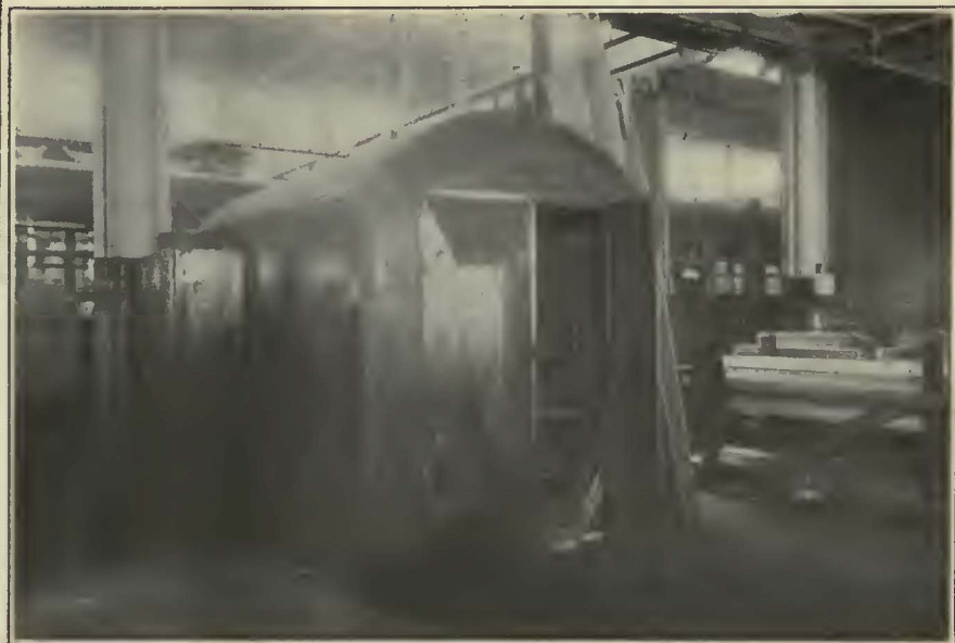
Sheet Iron Oven Installed in the Wood-Working Section of the Department of Street Railways, Detroit, for Keeping Wood Stock at a Temperature Suitable for Gluing
