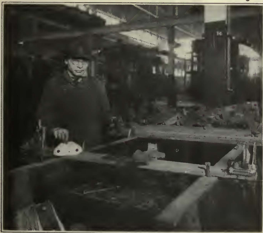
Installing a Canvas Pad at the Center Connection to the Brake Beam in the Shops of the Department of Street Railways, Detroit, Mich.
