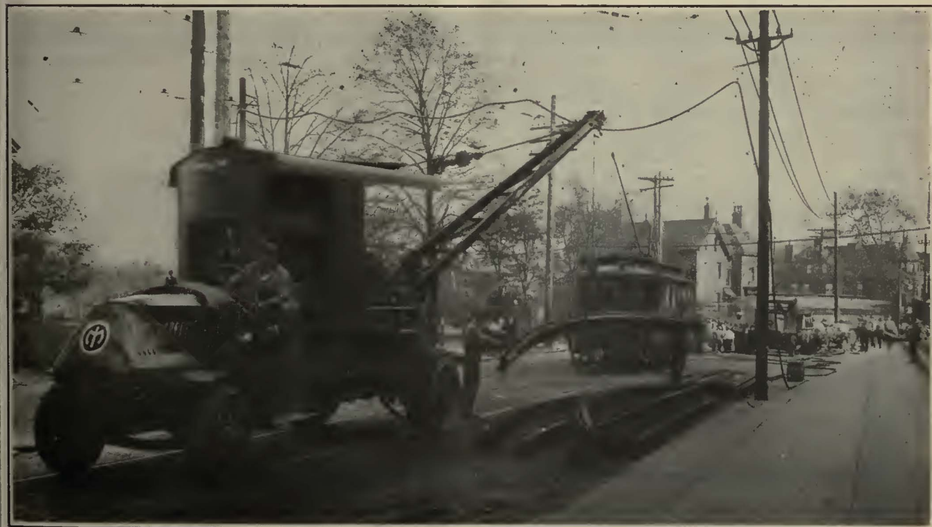
For Placing Rails in Position After They are Unloaded at the Side of the Street the New Cranes Are Found of Particular Convenience
