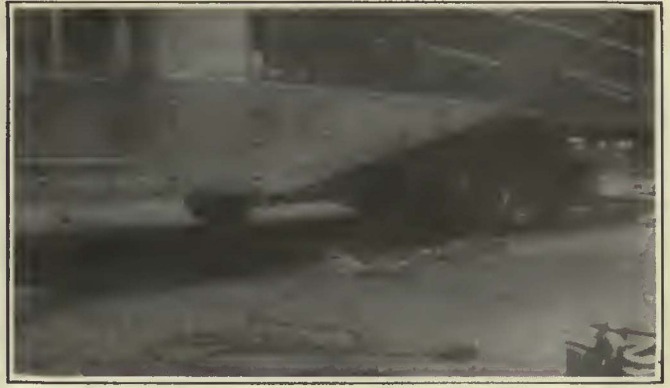
The Unsightliness of the Rusted Side Is Obviated Through the Use of Steel Plates Similar to the One Pictured Here
