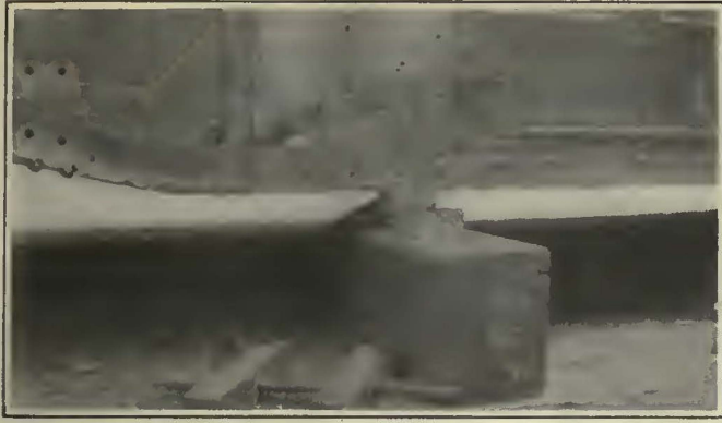
This Car Side Has Been Entirely Rusted Through by the Water Encountered in Operation
