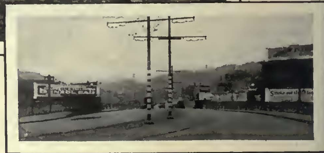
Scene of one of Cincinnati's more recent installations of Carey Elastite System of Track Insulation—Gilbert Ave., laid in 1924.
