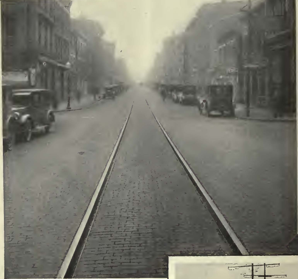
A section of Central Ave., Cincinnati, where Carey Elastite System of Track Insulation is used. Note the perfect condition of the paving where the wood blocks adjoin the rails. Yet this paving and these rails have carried a continual stream of heavy traffic since 1919.
