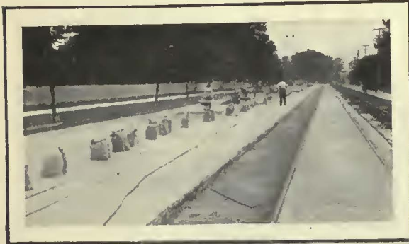
1926 view of Spring Grove Ave., Cincinnati, showing use of Carey Elastite System of Track Insulation where the pavement and rails adjoin.
