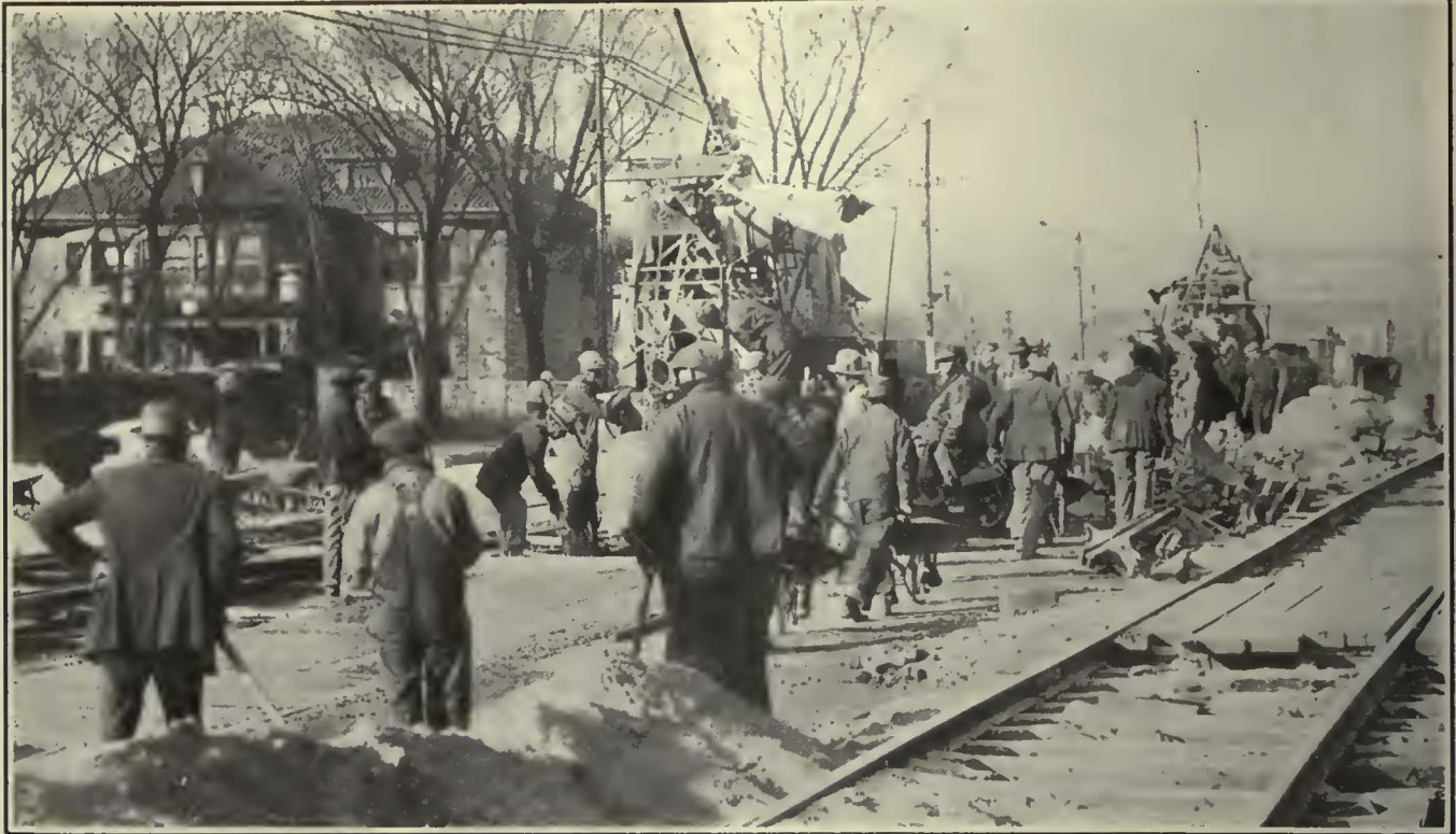
Putting on the Concrete Wearing Surface on Main Street, Kansas City. This Is Part of a Rush 8-Mile Reconstruction Program Completed Within Eight Weeks Following the Termination of Receivership Last October
