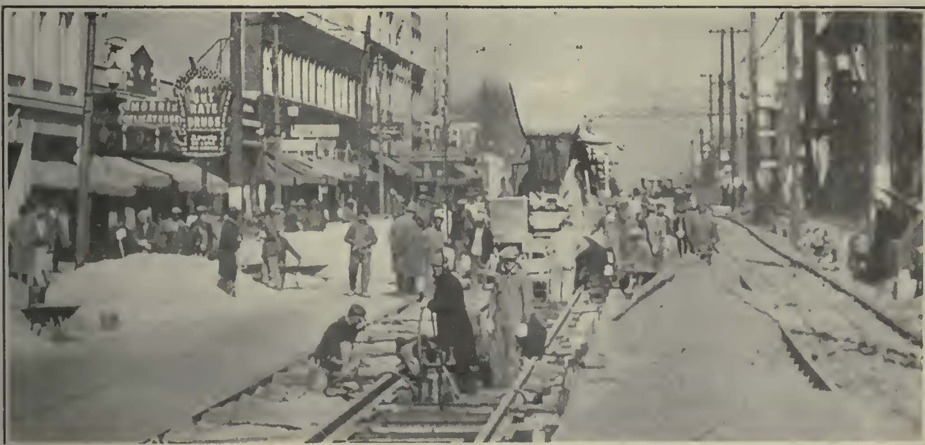
Part of the Initial Track Reconstruction Program in Progress on Troost Avenue, Kansas City. The Standard Construction Is 7-In. Tee-Rail on International Steel Ties Imbedded in a 14-In. Concrete Slab
