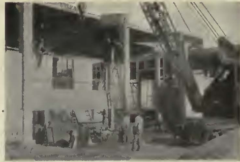
Placing wall slab, with window frame and sash, machine shop, Stockton, Calif.
