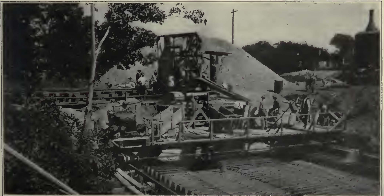
Mixing Plant at One End of the 400-Ft. Culvert Being Constructed Prior to the Erection of the New Car Station of Cleveland Railway on West 117th Street. A Ford-Driven 36-Ft. Bridge Carries the Mix and Other Materials to Any Point on the Job, Part of Which Extends Around a Curve
