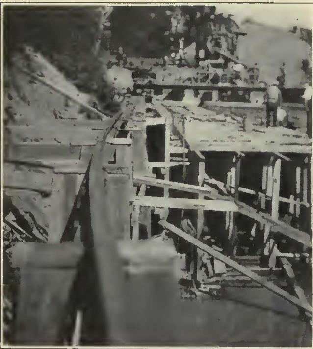
At the Point of Tangency on the 400-Ft. Runway Over the Culvert a Second Rail Is Used to Accommodate a Larger Wheel, Allowing Bridge to Swing Around Curve in Perfect Alignment
