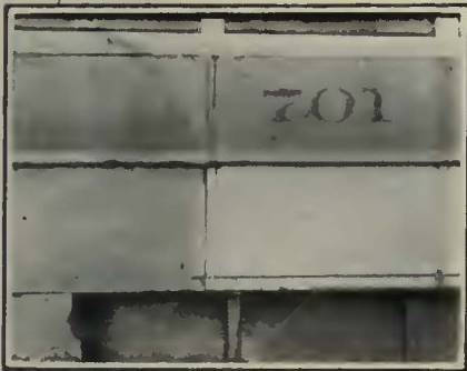
The Light Part of the Panel has Just Been Cleaned. The Remaining Part of the Car Is in Its Original Condition
