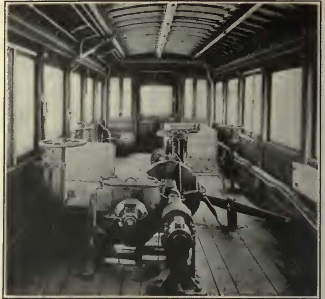
All Electrical Equipment, such as Resistors, Compressors, etc., Is Installed Inside the Car
