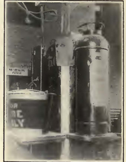
Fire Station Located on Central Posts in the Shops of the Grand Rapids Railway
