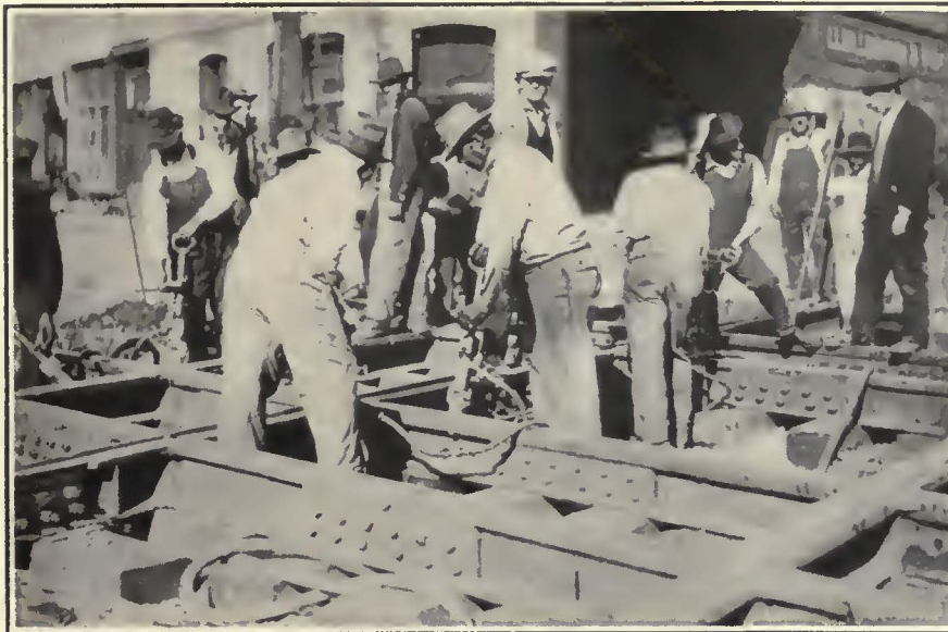
At Work with Air-Operated Tamping Tools on a Double-Track Crossing. The Air Used Is Furnished by the Portable Outfit Mounted on Bus Chassis
