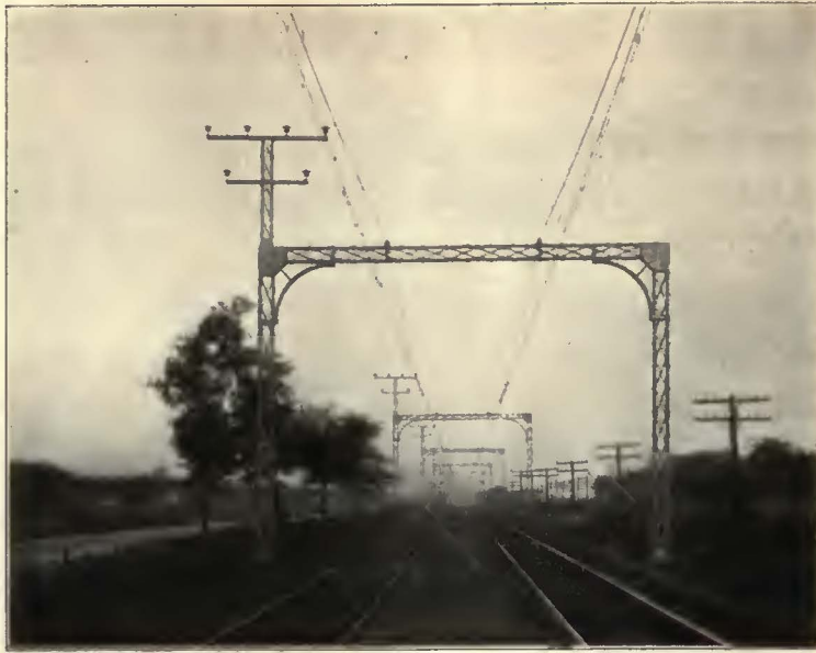
View of the "Ideal Mile", Chicago South Shore and South Bend Ry., showing Bates "Semi-Fabricated" overhead structures. Photograph used through courtesy of the Ohio Brass Co., who furnished catenary material.
