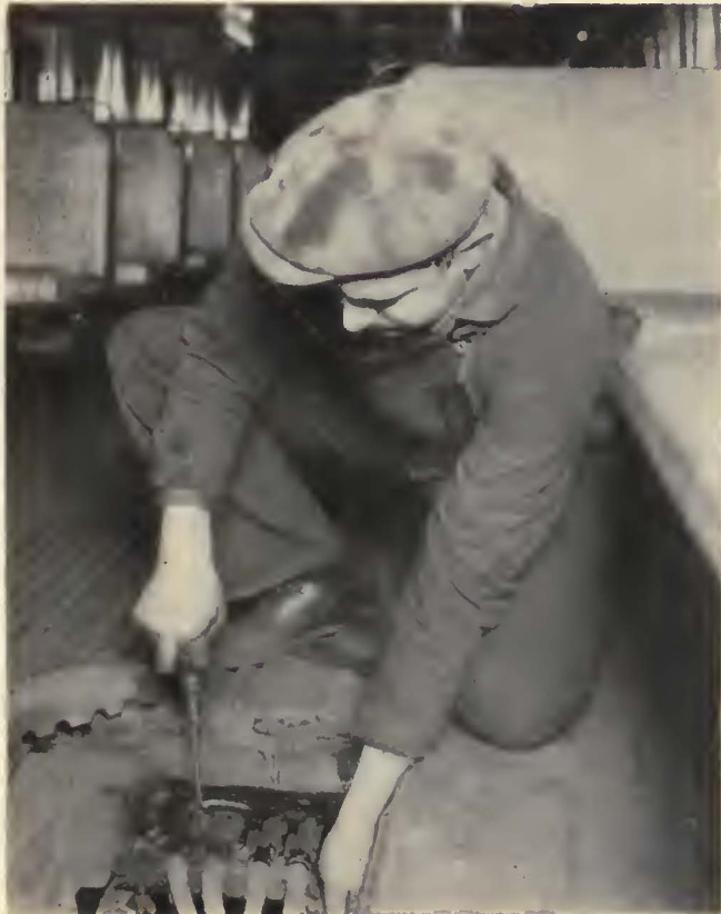
Motor lead junction boxes were inspected carefully and all connectors tightened
