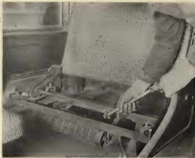
Heaters were blown out with compressed air and all supports, terminals and coils were tightened
