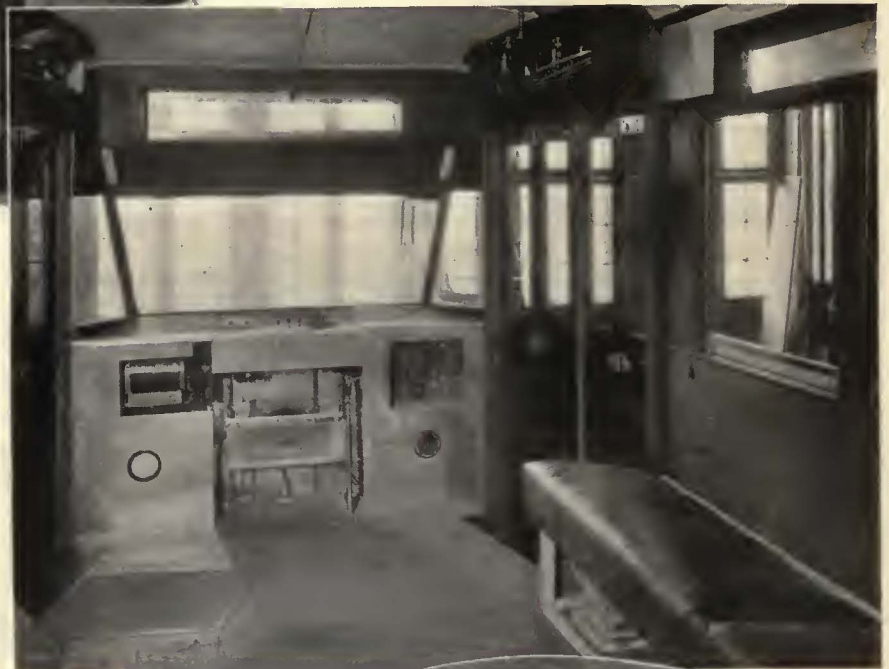
All switches and control apparatus are in cabinets at ends of car
