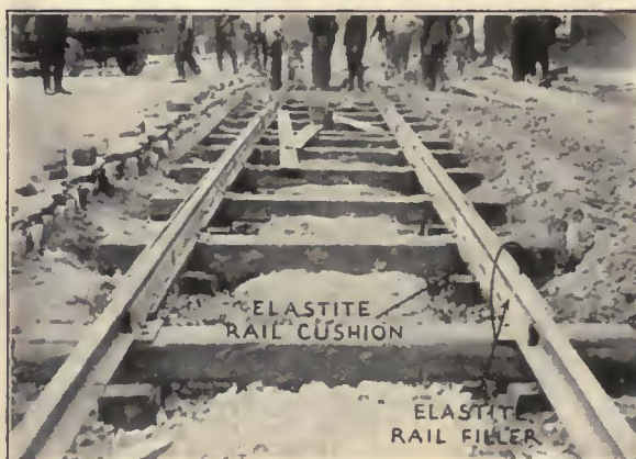
View of the Georgia Power Company Street Railway, on Hunter Street, Atlanta, Georgia. Note the interesting construction features, and the Carey Elastite System of Track Insulation in place.
