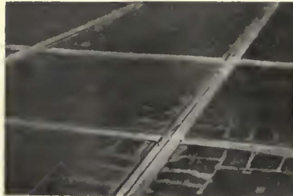
Built-up crossing which has been maintained in satisfactory operating condition by electric welding on the Market Street Railway
