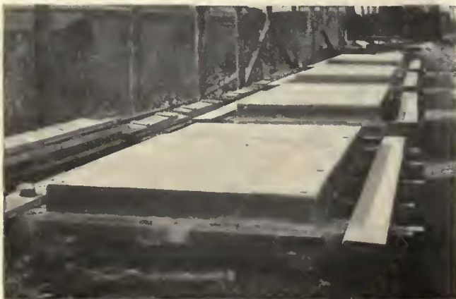
Precast slabs for loading platforms built by United Railways & Electric Company, Baltimore
