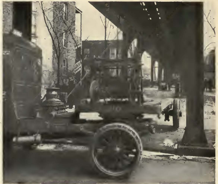
In pulling overhead cables with a winch truck, it is necessary to anchor the cable reel
