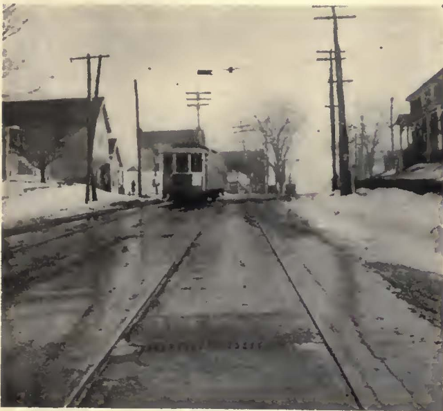
Asphalt paving with 8-in. concrete strip on each side of rail. Flangeway is made by means of template shown on preceding page
