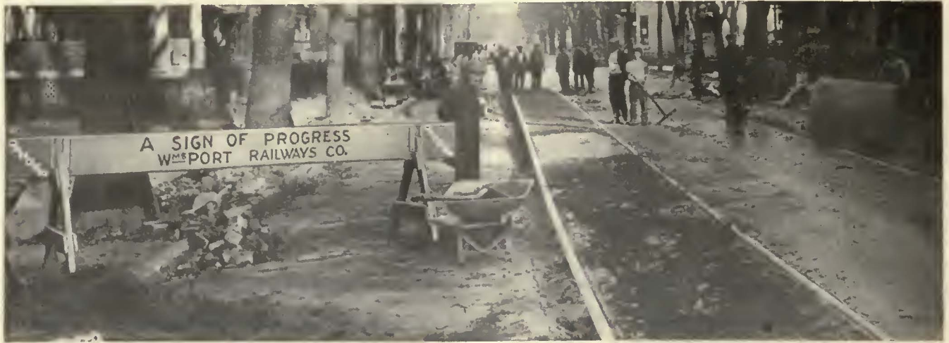
Part of the track reconstruction program under way following recommendations of the Williamsport Traction Committee that will extend over several years
