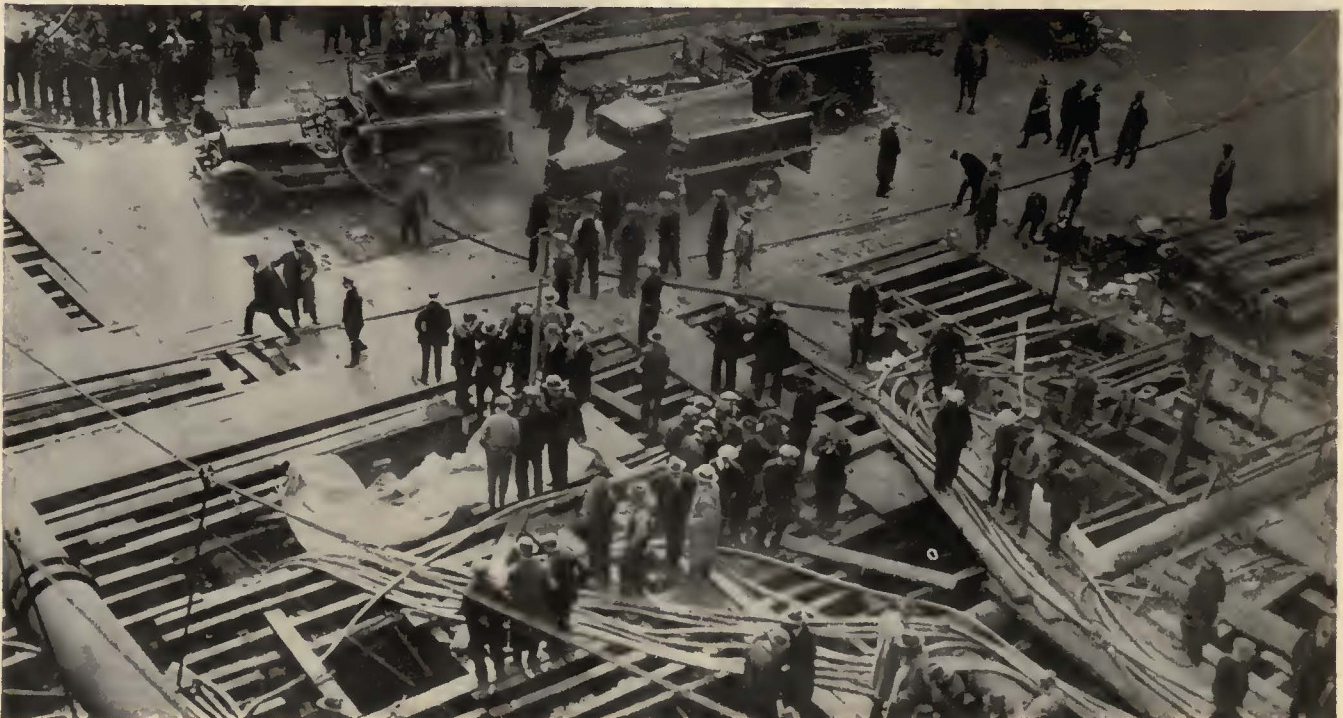
This view of the second fire shows great patches of planking torn up and temporary electric cables installed
