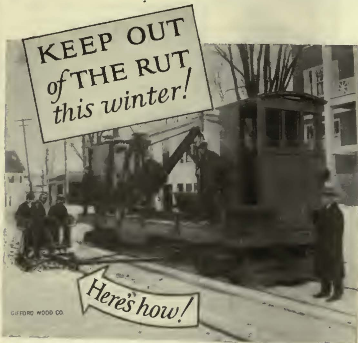
Gifford-Wood WAGESAVER Street Ice Leveler, operated from boom on derrick car, leveling ice on street outside of tracks. Cumberland Light and Power Co., Portland, Me.
