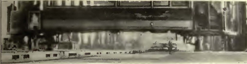
Hydraulic jacks on each side of the transfer table lift cars very rapidly for truck exchange in London
