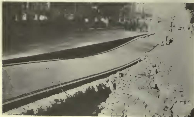
Section of Omaha track undermined by water from broken main
