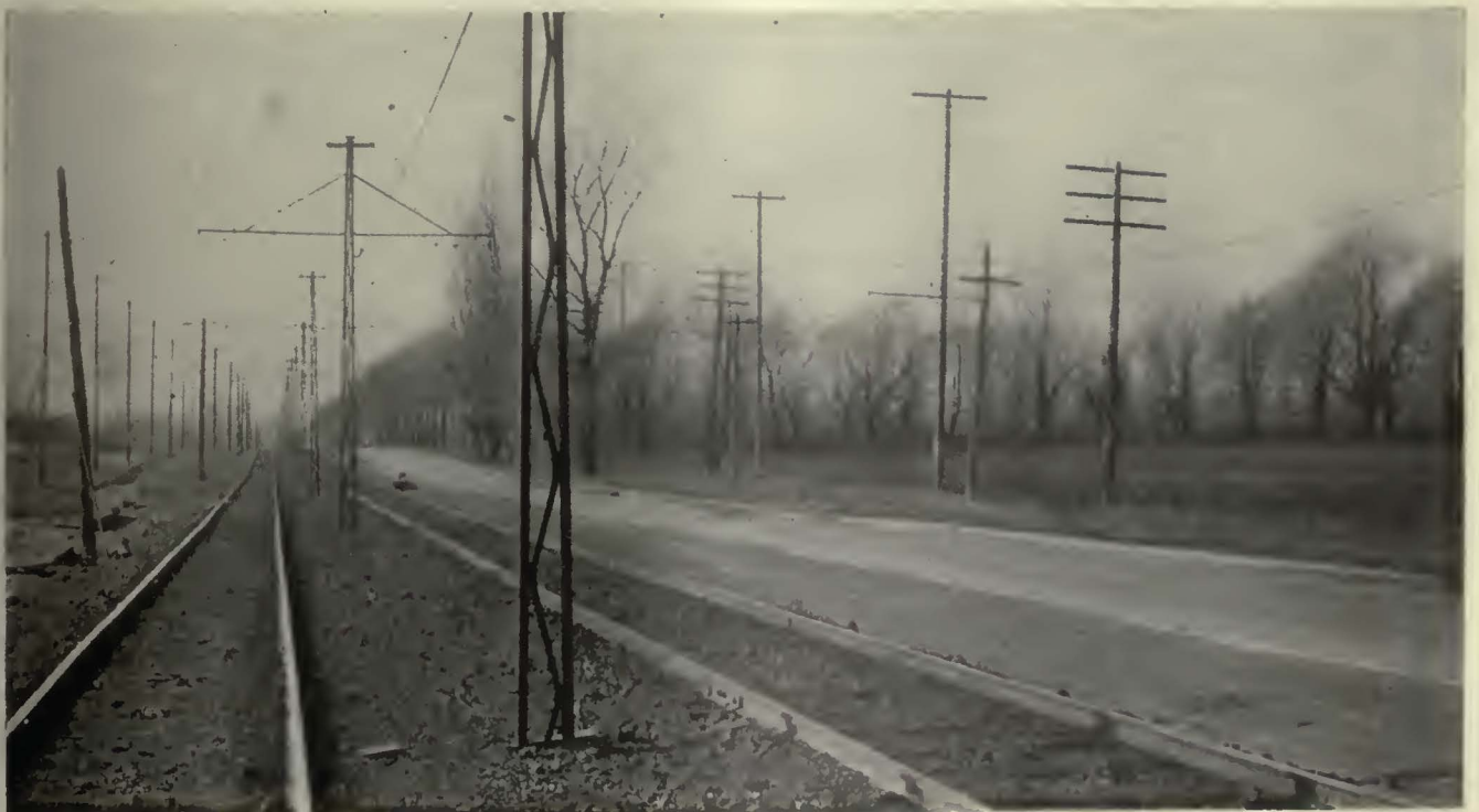
Appearance of the tracks and overhead construction on the 22-ft. island located in the center of the East Lake Road improvement
