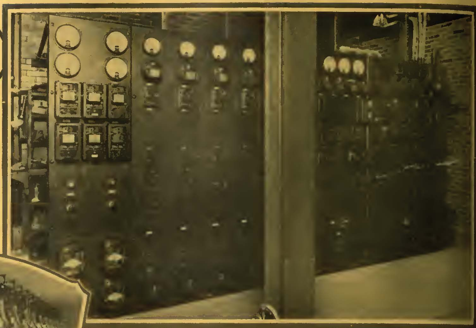
Automatic Railway Switchboard, Installed by the Indianapolis Street Railway Company →
