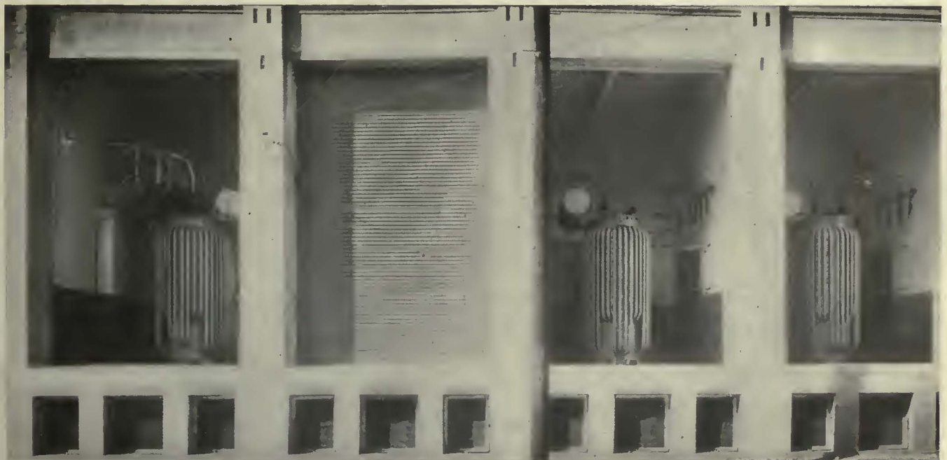
Transformers are installed in fireproof compartments with forced ventilation, opening only to the outside
