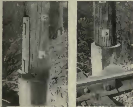
Two views of the completed butt, showing how the pole is bolted to the projecting tongues
