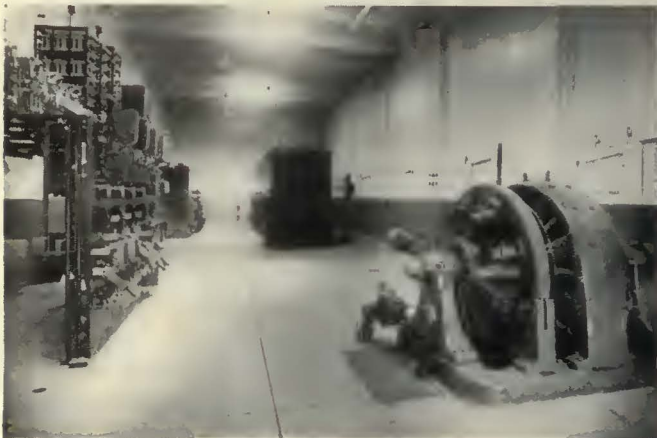
Interior view of the Principe substation showing the positive d.c. board, equipment for the 4,000 and 13,200-volt trucks and the 1,000-kw. converter
