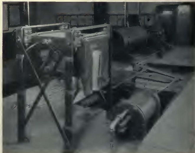
The air-brake equipment is mounted upon the floor of the car and can be inspected easily
