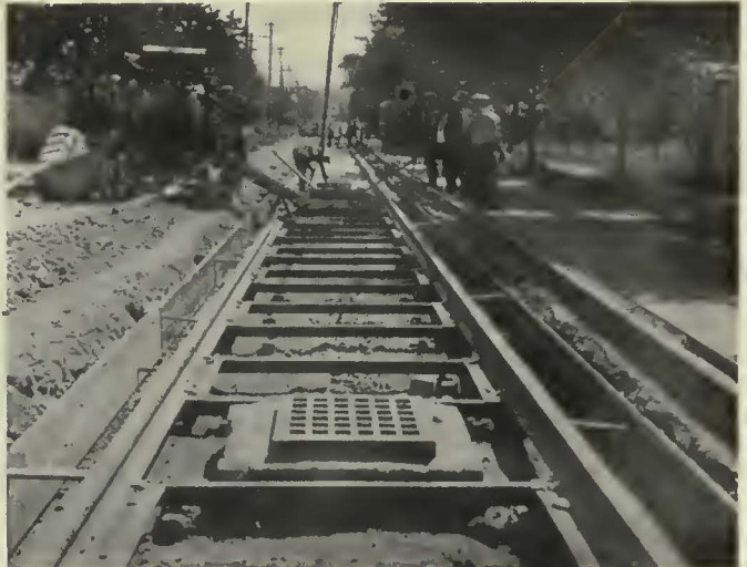
Another stretch of reconstruction work where traffic could be rerouted shows progress of the work. International steel ties were used on this job
