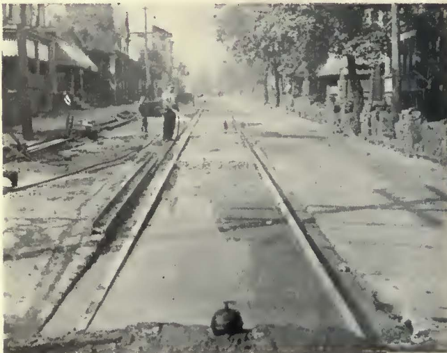
Curing the concrete on one of the stretches of new track constructed by the Altoona & Logan Valley Electric Railway in its 1927 program
