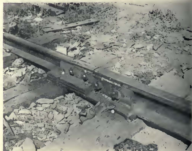
Where compromise joints were necessary in changing from one section of rail to another steel sole plates were welded to the rails, with filler plates to give a firm footing to the low rail
