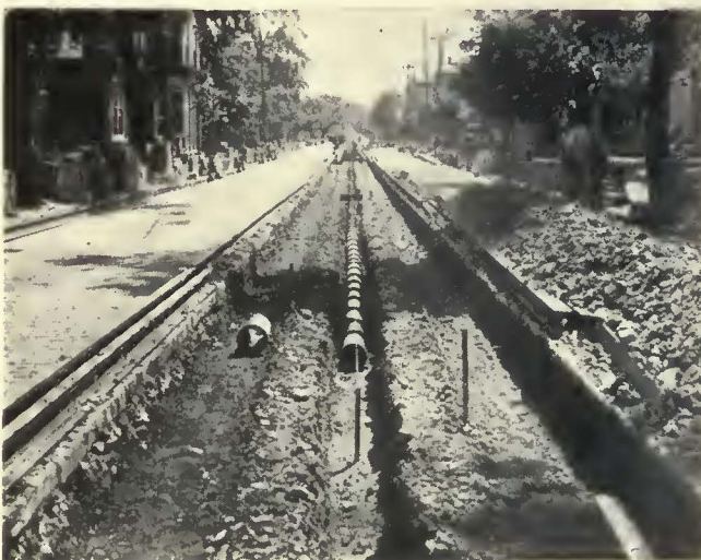
On account of the marshy soil in Altoona tile drains were laid under all of the tracks. This view shows a standard type of drain under the center of the track
