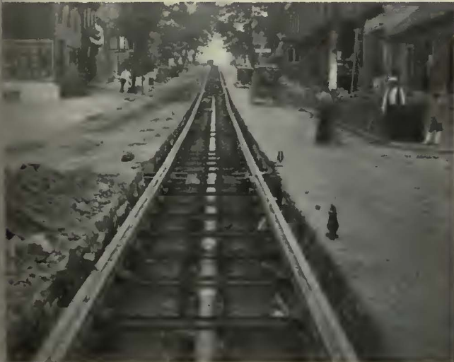
Where it was possible to reroute traffic steel ties were used in the reconstruction work. This view, taken on Allegheny Street, Hollidaysburg, shows the use of Dayton mechanical ties
