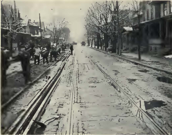
One of the stretches of track that was rehabilitated. In this view the temporary track is being laid alongside preparatory to tearing out the old track so that the service will not be interrupted
