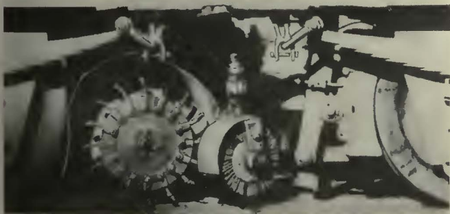
A work car cleans out the track groove and brushes the dirt away on the Rome Municipal Tramways. It also flushes the track. The upper view shows the complete car, the lower view shows the digging tool and rotary brush on a large scale
