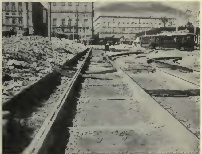
Track construction in downtown Naples. The timbers shown are simply to protect the fresh concrete and will be taken away after that has set
