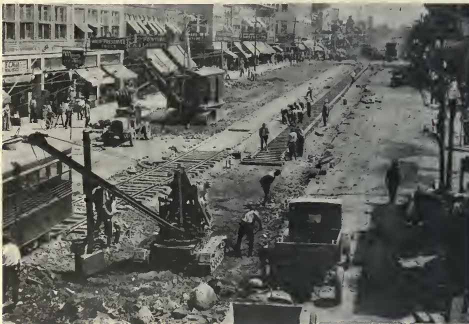
The Saginaw Street improvement included the complete reconstruction of 1½ miles of double track
