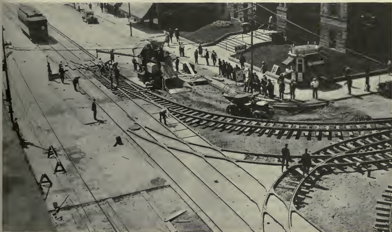
Street car service was uninterrupted during the construction. One track was poured at a time and operation continued on the other track
