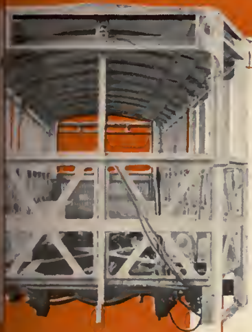
Front end view of Versare body framework. Note the rigid channelling and girder trusses.
