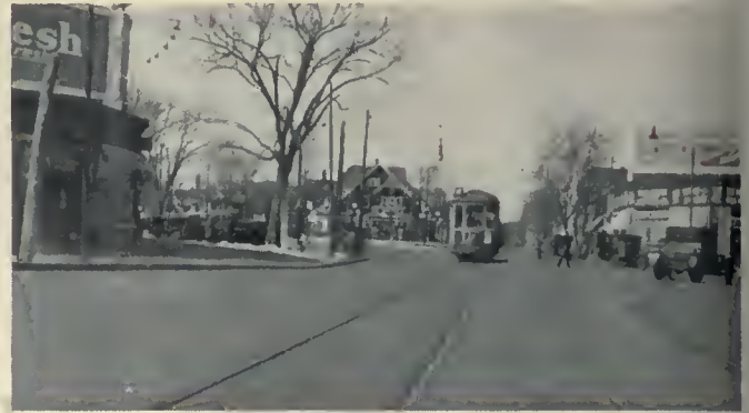
Double track installed on Belmont Avenue to speed up the service on a heavy traffic line
