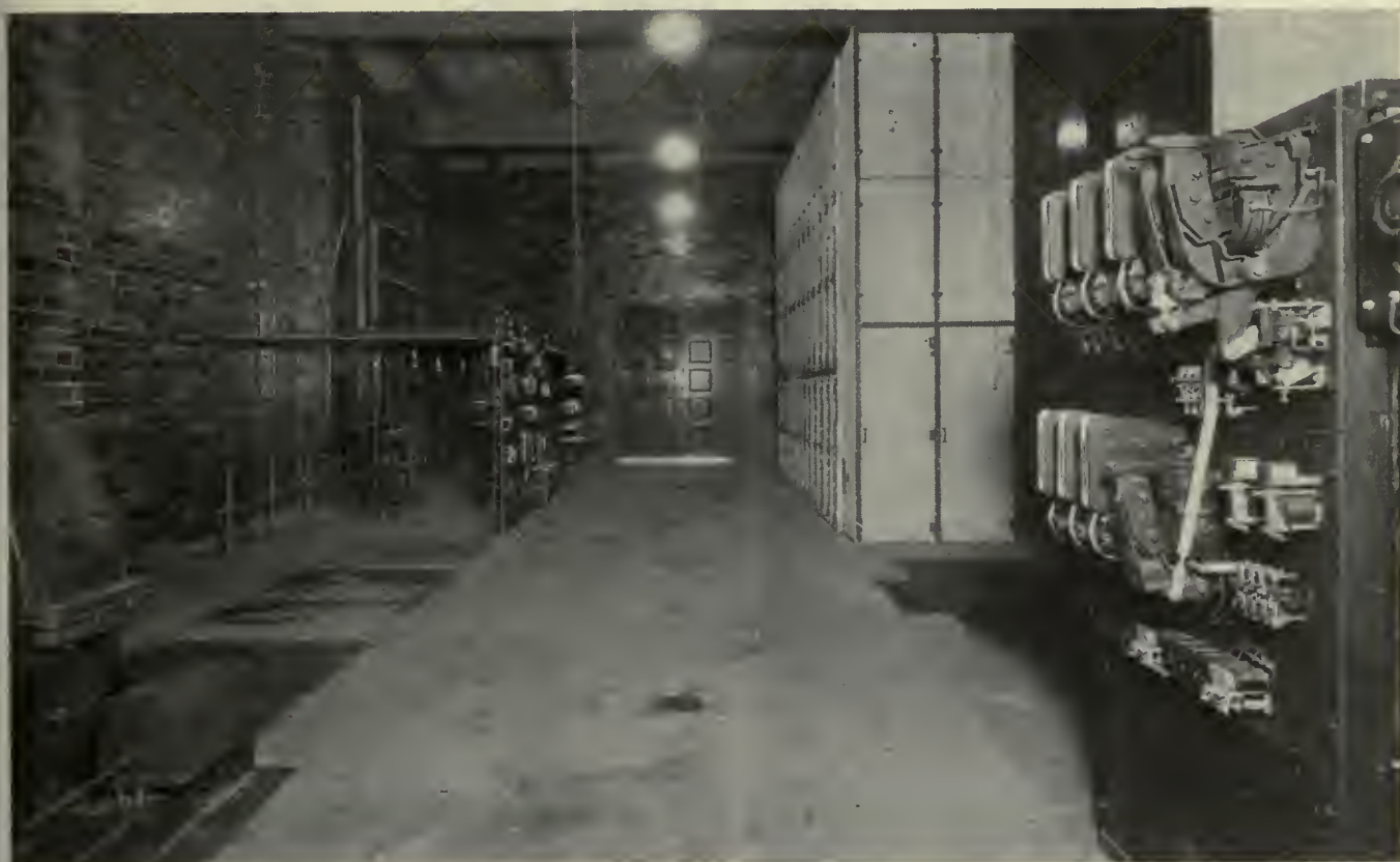
Interior of Colerain substation, showing typical arrangement of station equipment, provision for additional unit and "Deceleco" bus cell construction. The transformer is located behind the switchboard at the right
