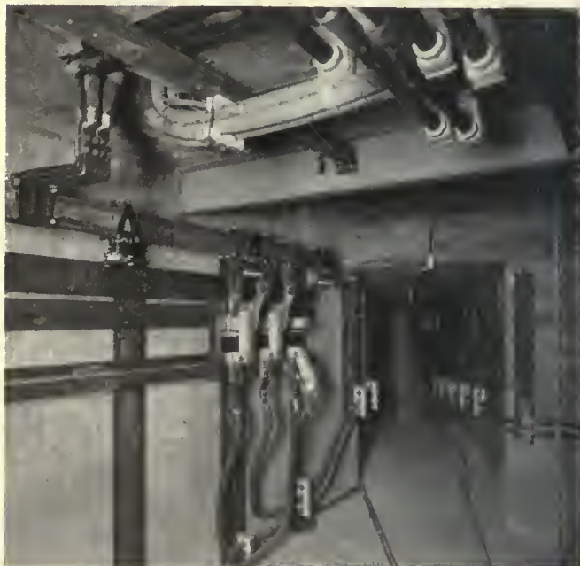
Basement view of Cincinnati substation showing negative bus structure and method of carrying feeder lines to street
