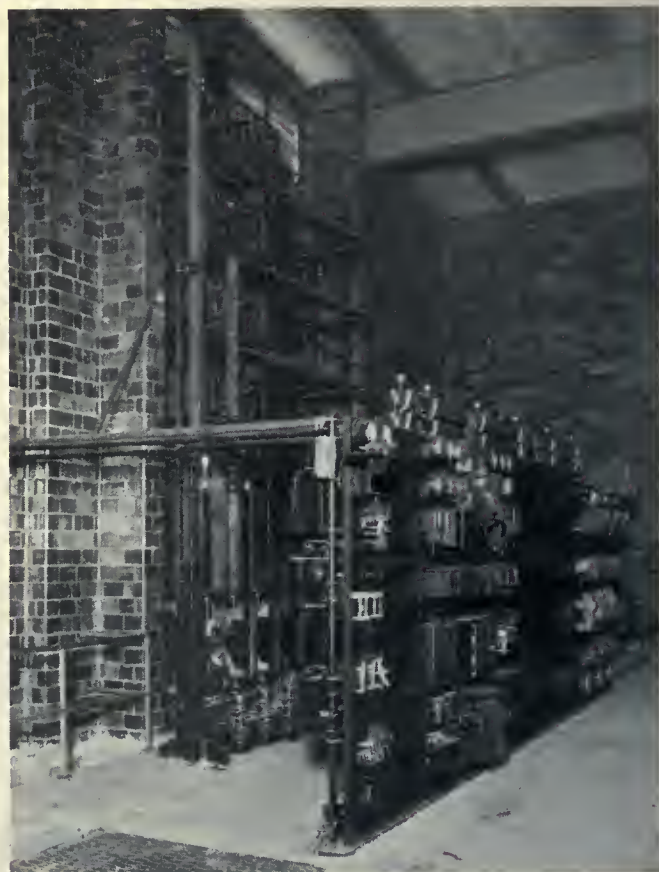
Interior view of station showing load-shifting resistor mounting, floor grating and side wall louver near ceiling for ventilation
