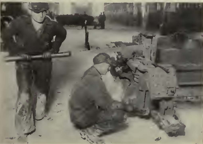
Bolts are installed under journal boxes quickly by means of a lever attachment that compresses the spring between the truck frame and the top of the journal box
