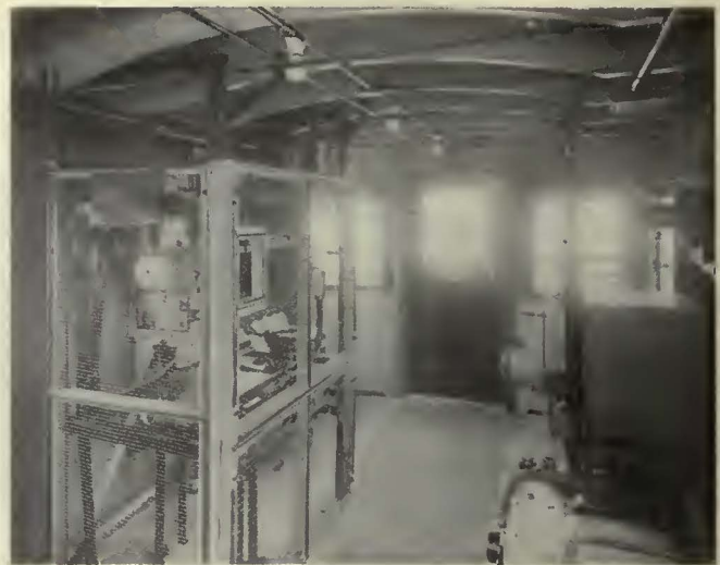
Interior of the locomotive. As a safety precaution, the control apparatus is inclosed in a wire cage
