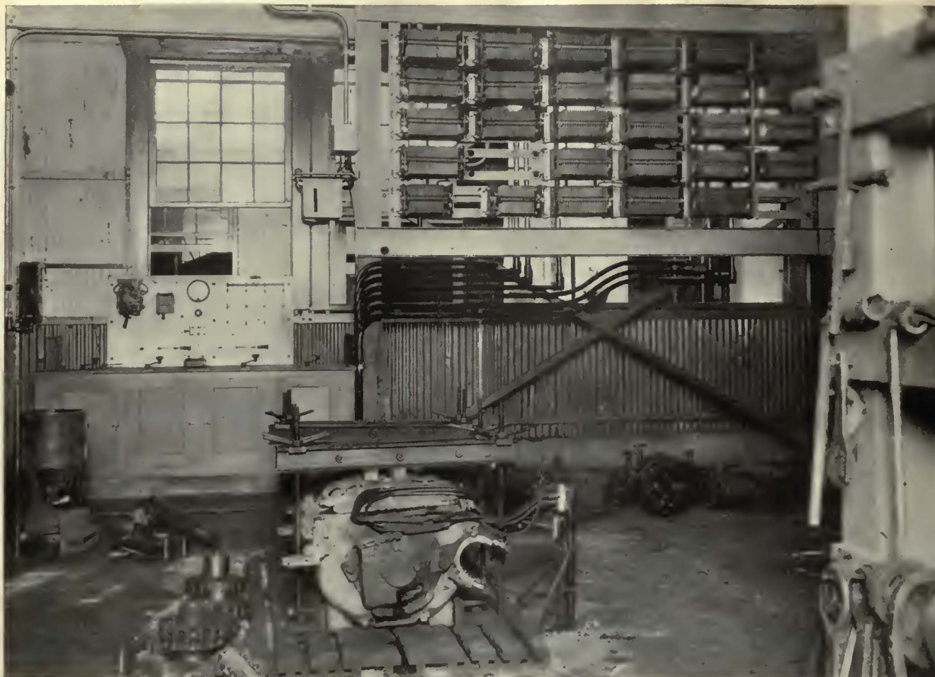
The motors under test are shown in the foreground and the switchboard and load rheostat in the background
