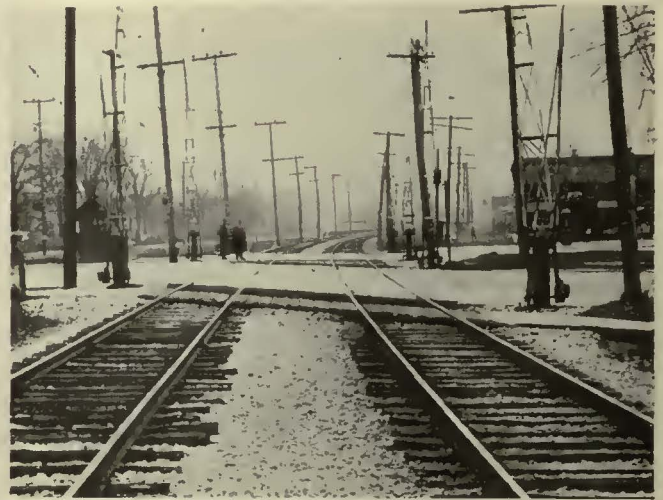
The left-hand or northbound track was raised 14 in. to eliminate double bump in highway crossing
