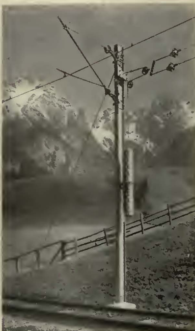
Standard steel pole with tension take-up weights between Leogang and Hochfilzen on the Wörgl-Saalfelden route, Austrian State Railways
