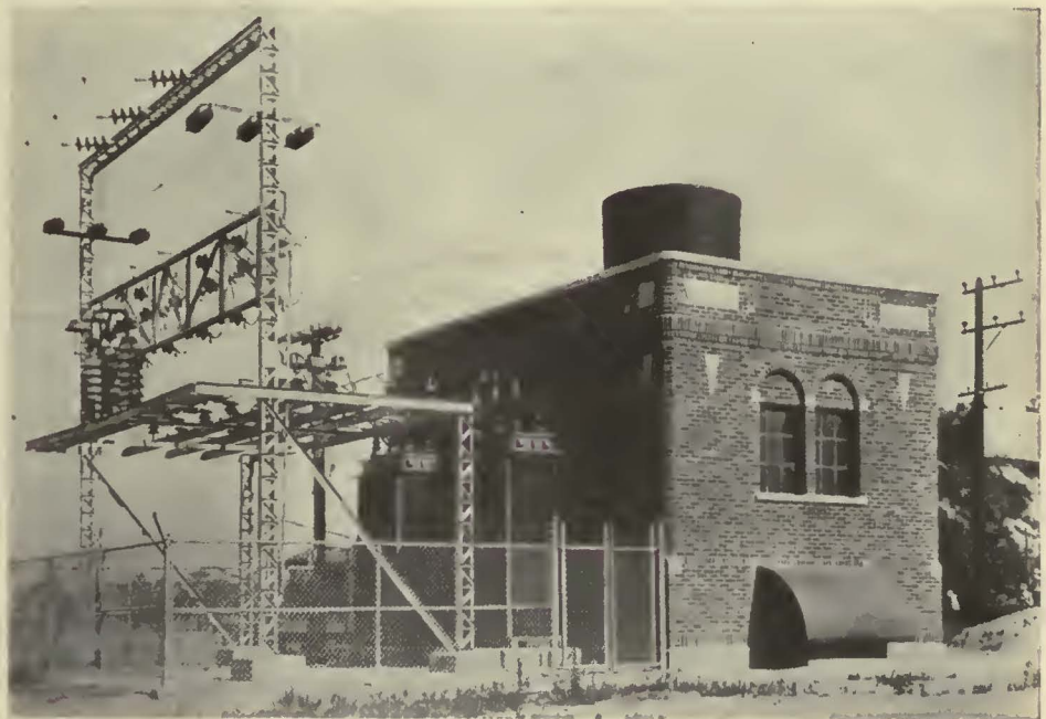
One of the substations, showing the high-tension equipment and the hood for protecting the air inlet
