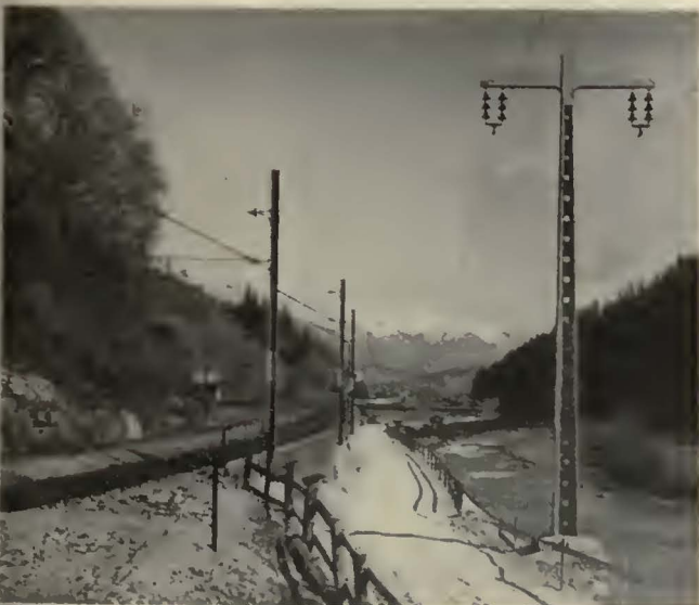
Perforated concrete poles used by the Austrian State Railways for transmission line between Hopfgarten and Soll-Lenkental on the Wörgl-Saalfelden route
