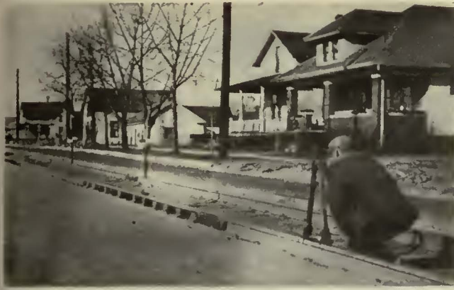
The track was surfaced and aligned by means of a Buff Railign instrument
