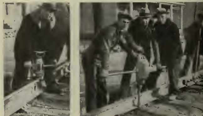
Holes were drilled with an electric drill and the screw spikes placed with a spike driver
