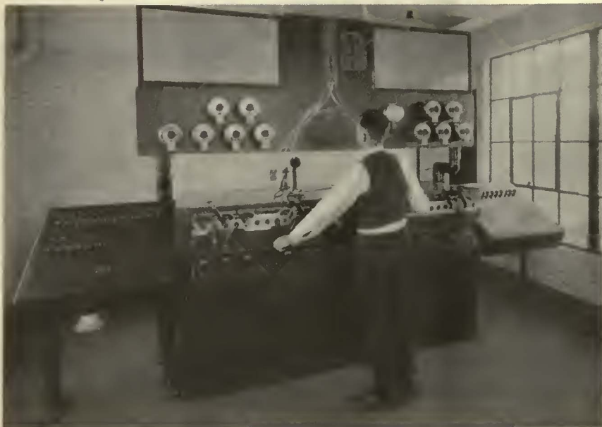
Interlocking machine at yard portal for switches on the main track. Note the control panel at each end for controlling yard switches, the track model showing the main track layout and framed charts on each end showing the respective yard layouts
