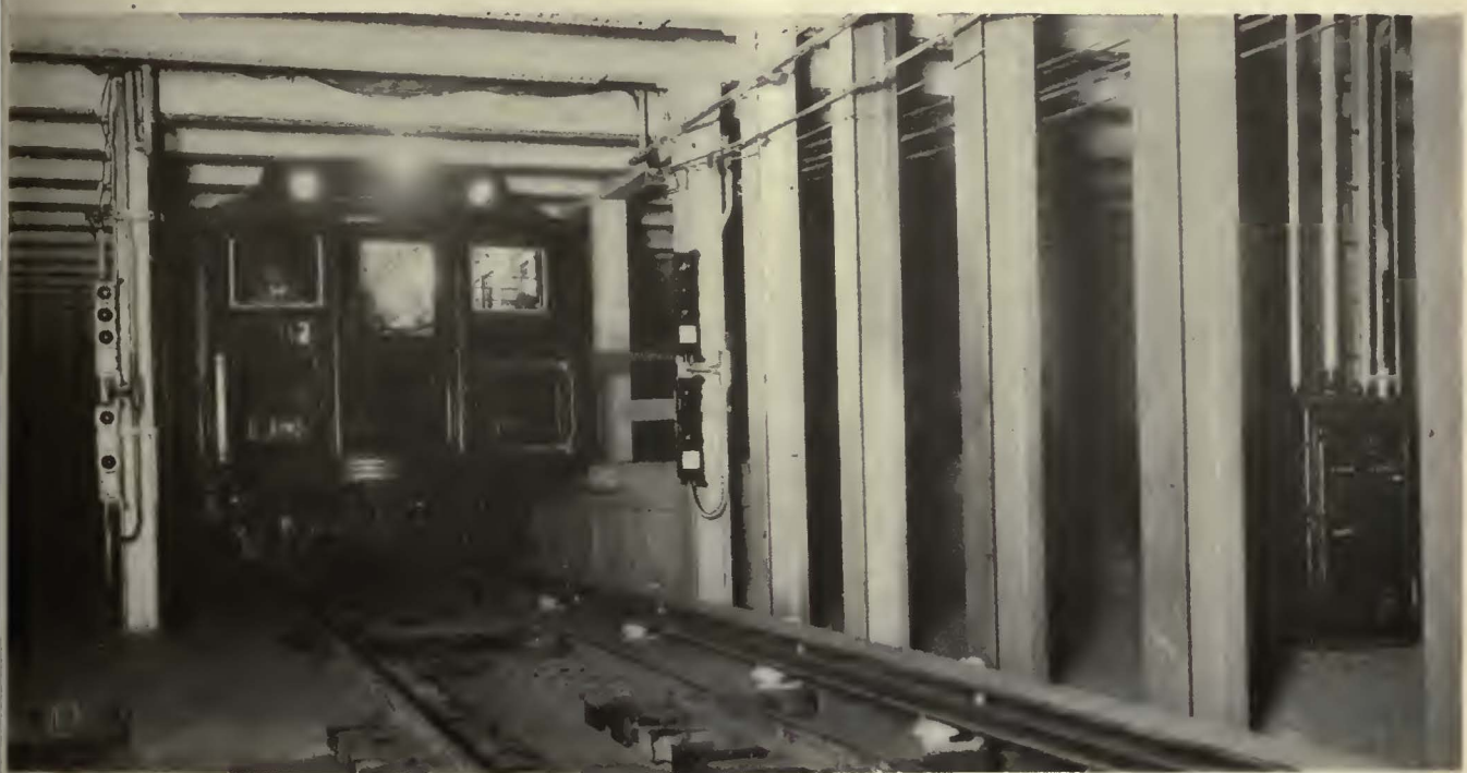
Signal location at Olney Avenue, showing the conduit run and the relative location of signals. Note the double case at the right and the method of running air line across track
