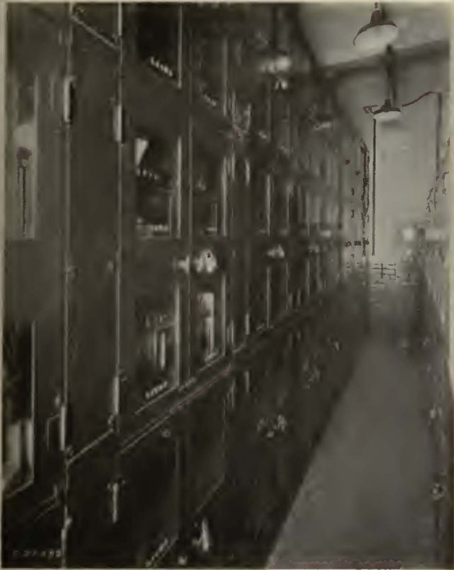
Three tiers of tower relay cabinets installed at the Olney station interlocking plant
