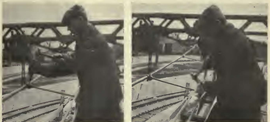
At left—The messenger end of the curve hanger is clamped securely to the messenger wire. At right—The intermediate wire is held in the curve hanger by peening-over a lip on the top of the clamp
