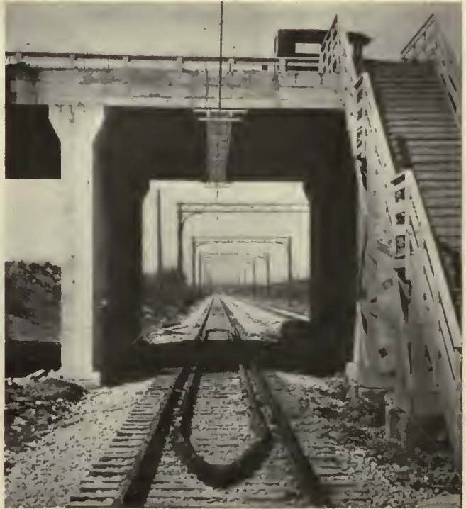
Catenary construction was used on all open-track main line of the Rochester rapid transit line
