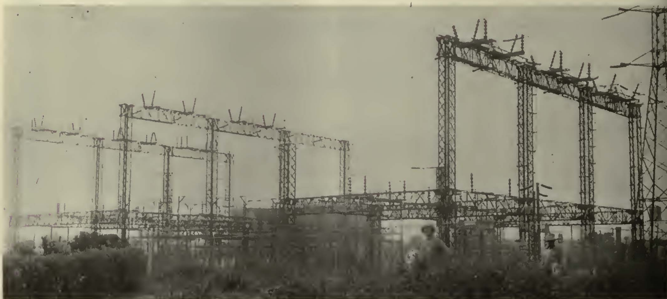
The high-tension structure carries the 132,000-volt line air circuit breakers, choke coils and lightning arresters
