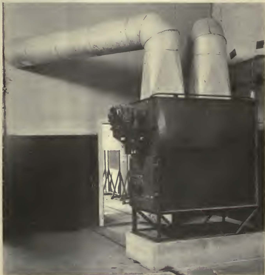
Blower used to force air through the paint room
