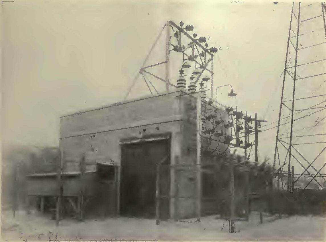
Exterior of Nemahbin rectifier substation, showing at left the sheet-iron housing for load-shifting resistors
