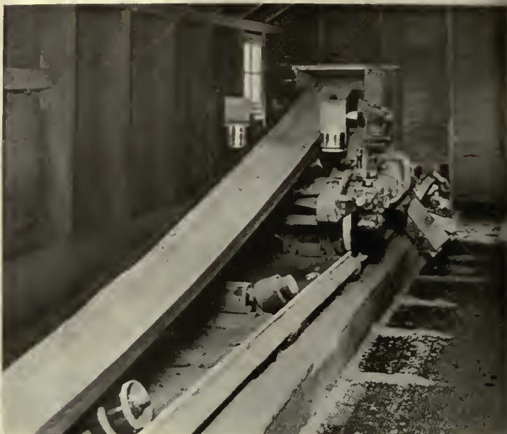
The dried sand is conveyed to the top of the sand storage bin where it is screened after leaving the belt. It then passes into the storage bins below
