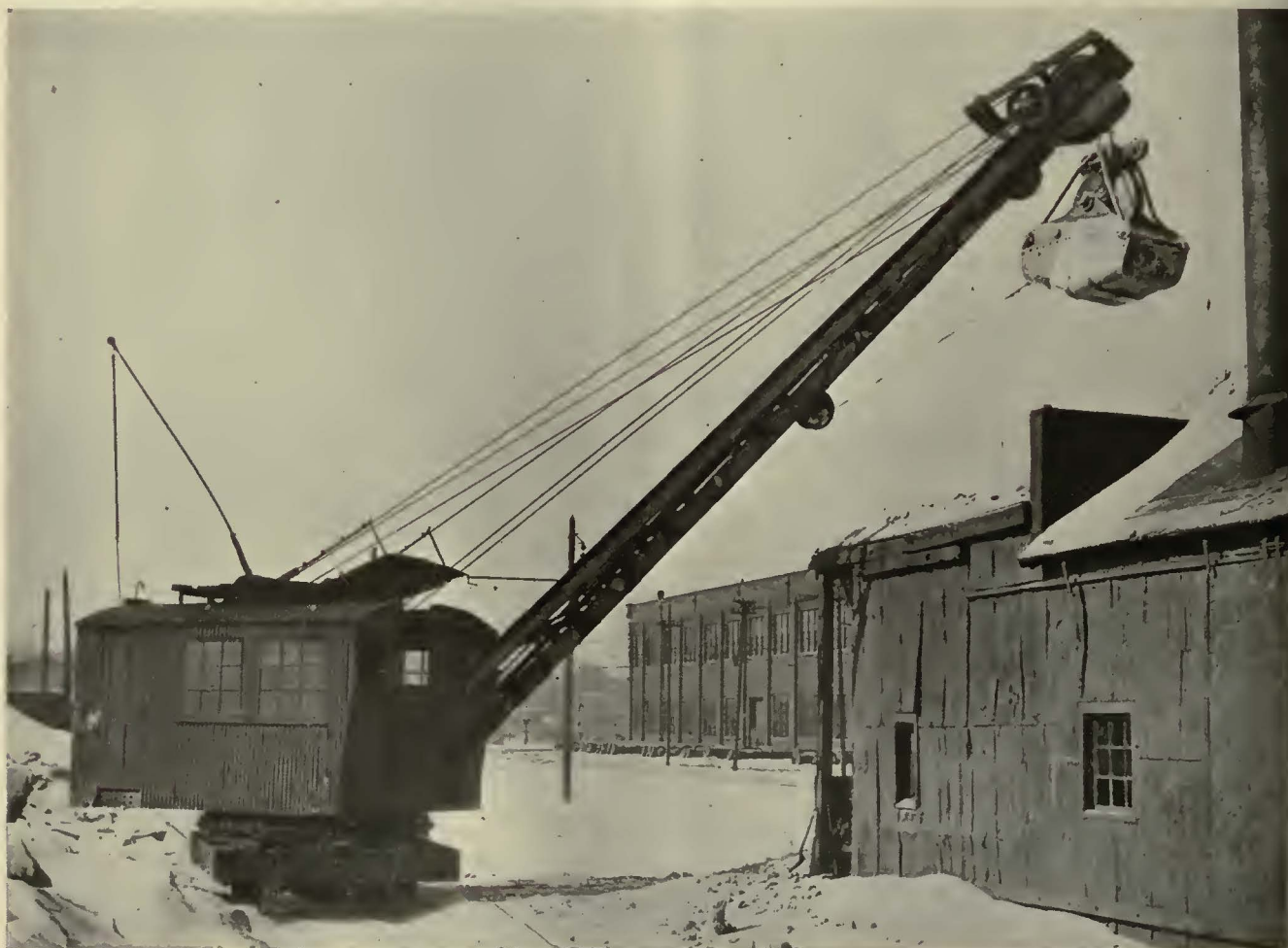
An electric crane equipped with a 1-yd. bucket loads wet sand into the 100-yd. capacity hopper
