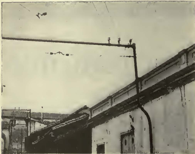
A contact wire does not have long life when only a few pull-overs are placed to support a curve. Excessive wear develops at the ear joints
