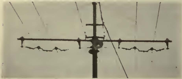
The secondary insulation between the positive and negative wires is so low it forms a drip point. The collection of sediment and eventual leakage of current and burning may be expected on the surface of the insulators
