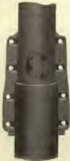
"H" Clamp Reinforcing Corroded Swaged Joint
