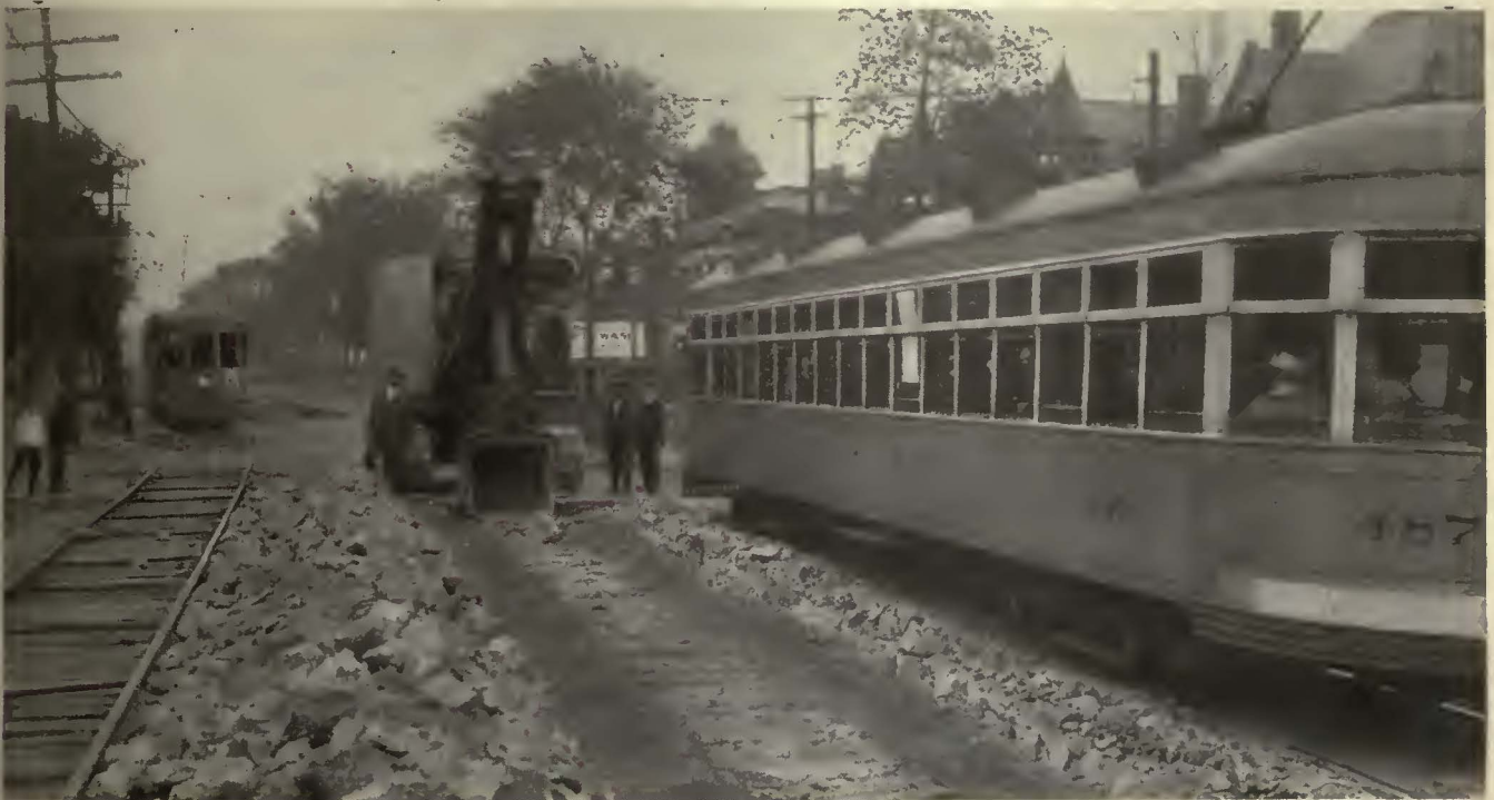
Tearing up old track without interference to car service which continued uninterrupted in both directions
