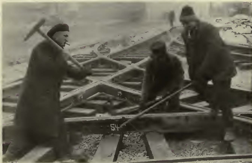
Using the tie nipper while spiking special work in Cleveland. By its use one man out of the crew of four is eliminated
