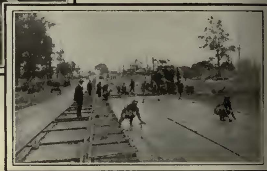
Photograph below shows laying and finishing concrete 12 in. deep on double-track construction job, in which Bethlehem No. 3 Steel Ties were used.
