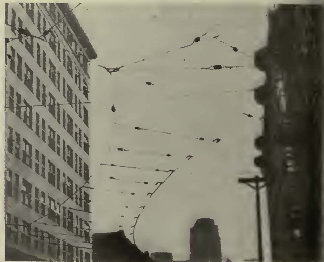
This curve is supported with the proper number of insulators. Note the double insulation in the pull-over wires
