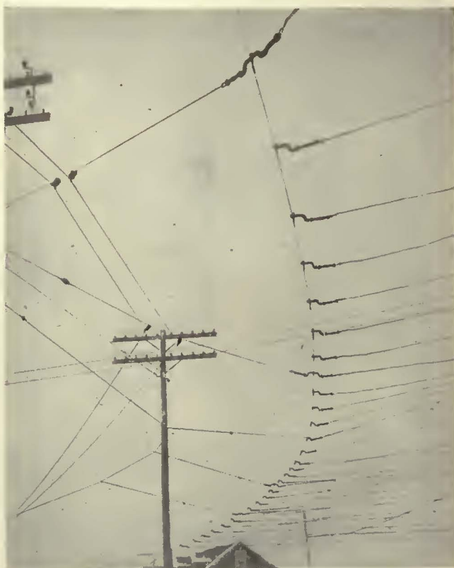
Too many pull-overs form a rigid overhead system. Usually it is impossible to maintain sufficient tension in the pull-over wires to prevent tilting of the fittings and side-swiping of the ears
