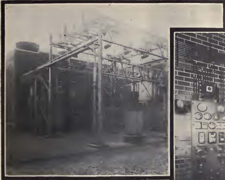
Maple Substation, Pittsburgh Railways Co.
