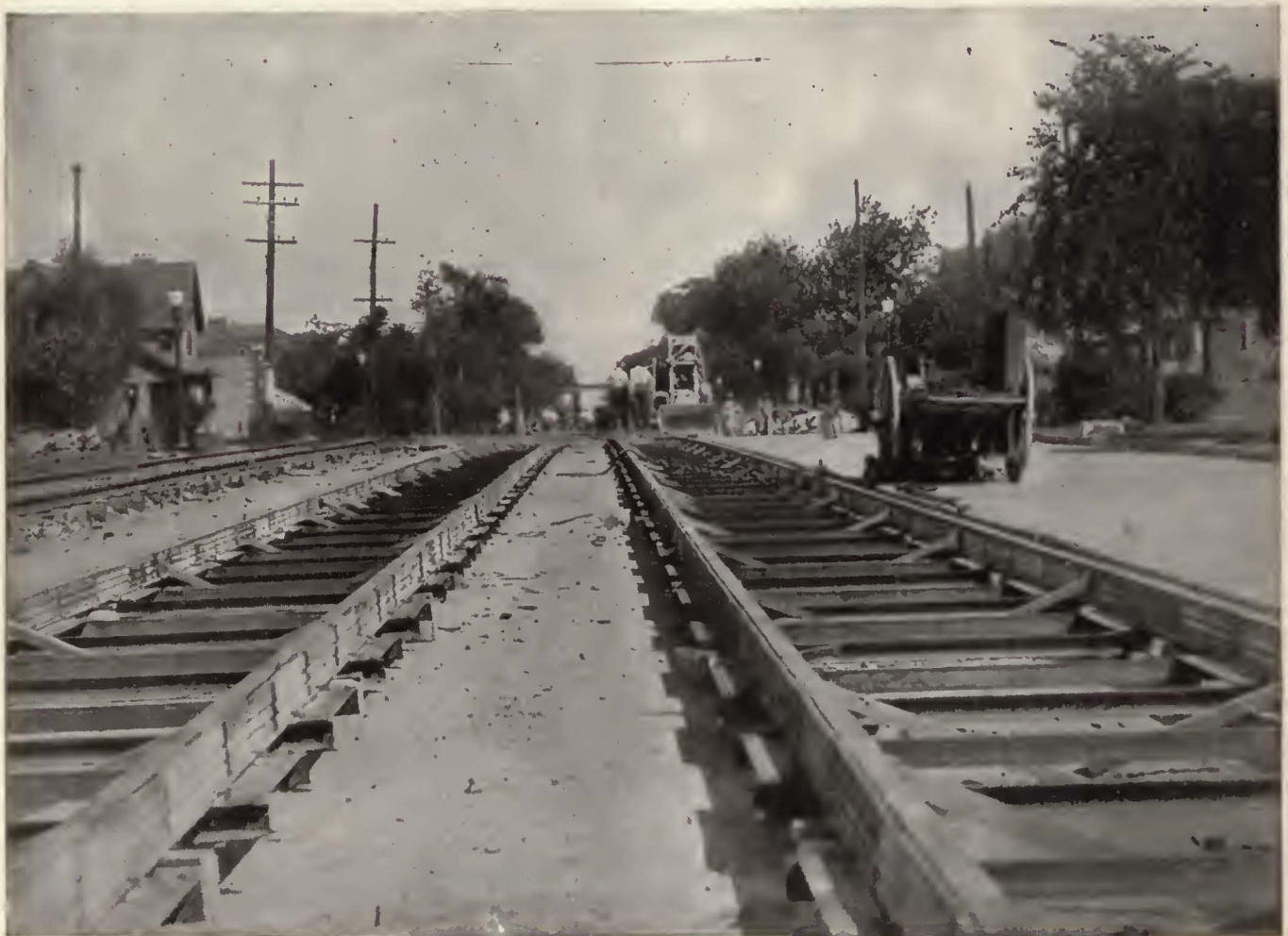
S HOWING the application of Carey Elastite System of Track Insulation on the Hydro-Electric Railway lines, at Windsor, Ontario, Canada.
