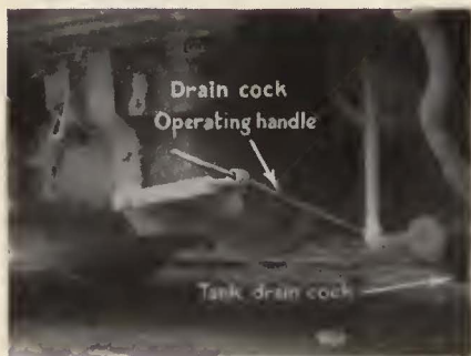
Since this operating rod has been in use all tanks are kept drained
