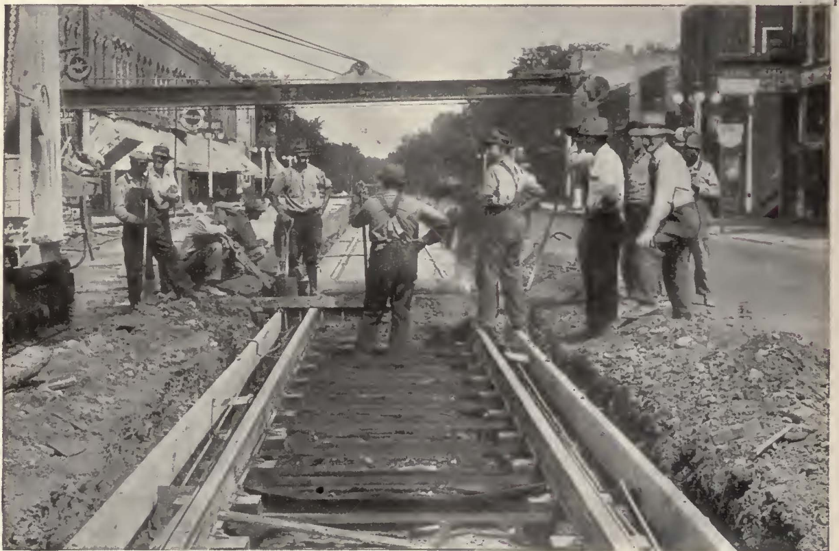
Showing the application of Carey Elastite System of Track Insulation on the Northern States Power Company's lines through Eau Claire, Wisconsin.
