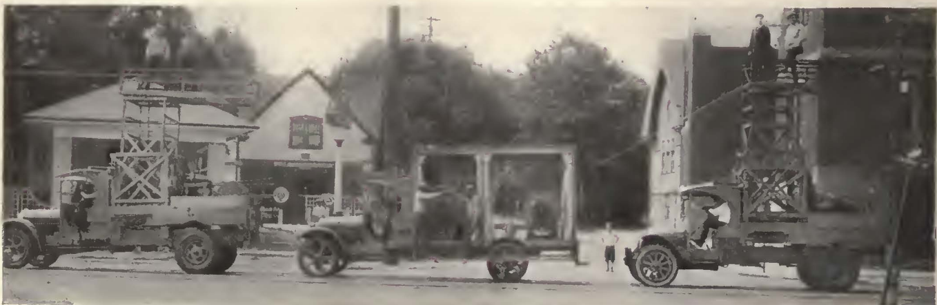
Use of this double-reel truck has facilitated the process of stringing trolley wire at Cleveland
