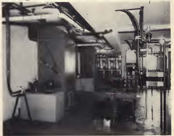
In the basement are located the recoler, the reactors, the negative bus and the house transformers. The reactors shown in the foreground are to eliminate telephone interference
