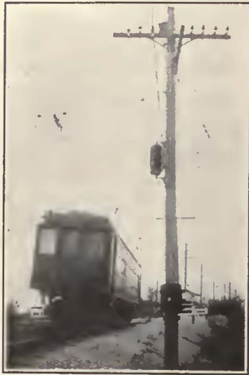
NACHOD rear protection 3-indication color light signals protect the fast and frequent movements on this progressive and high-speed interurban.
