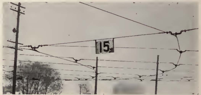
Adaptation of a double track curve for bow collection. Note that the hangers are inverted so that no part of the overhead projects beneath the plane of the contact wire
