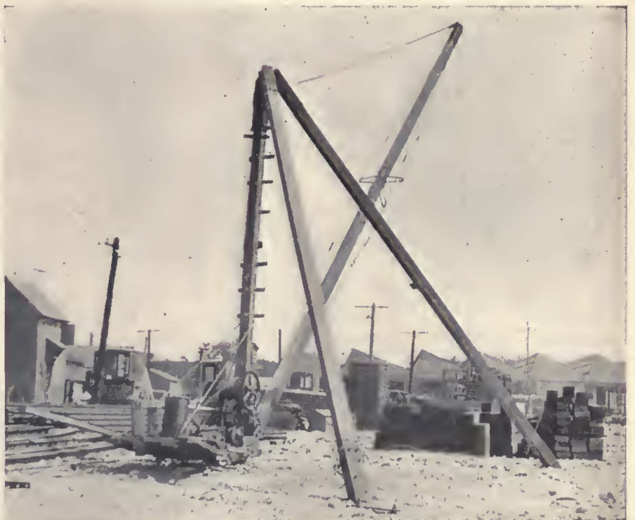
Stationary crane used in storage yard of the Virginia Electric & Power Company for handling materials resulted in a considerable saving in labor expenses, as well as a reduction in the number of accidents
