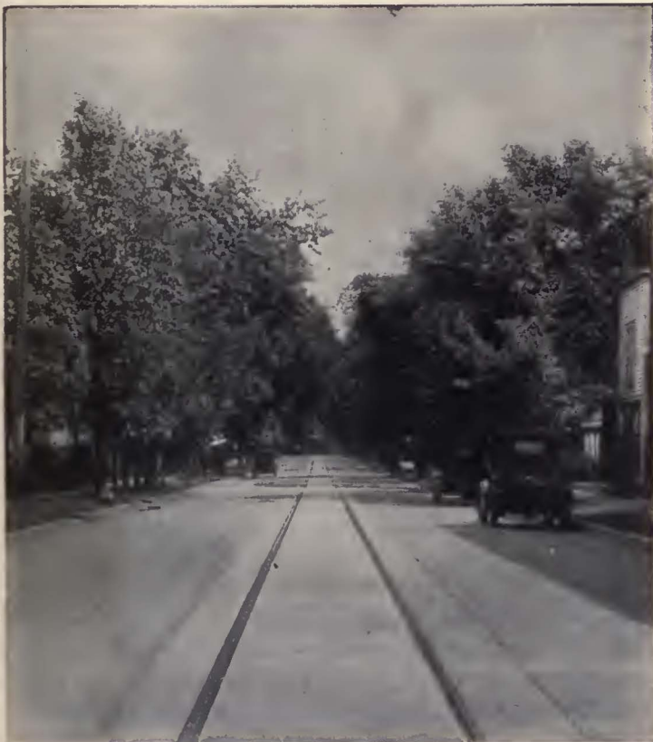
The completed installation—Carey Elastite System of Track Insulation, used in connection with a standard 85-pound A.S.C.E. T-Rail and a roadway of concrete.
