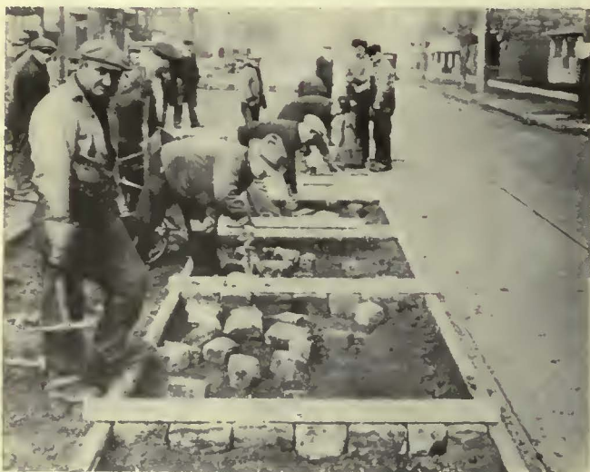
When paving with granite blocks the Cleveland Railway uses straight edges to insure level surface
