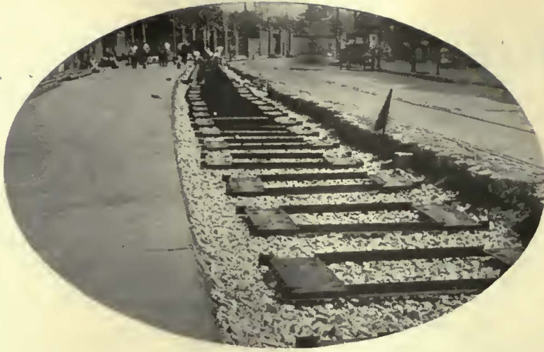
International steel Twin Ties spaced 6 ft. center to center were laid on a 3-in. layer of broken stone
