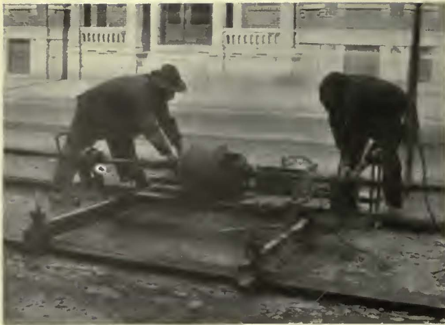
Penetration of the grout was assured by use of a revolving vibrator placed longitudinally between the rails
