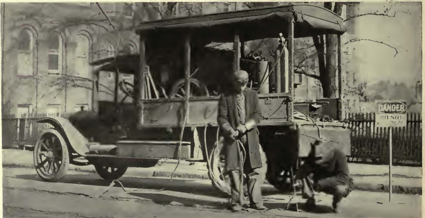
A complete electric welding set and an oxy-acetylene cutting equipment are mounted together on a 1-ton White truck by the Georgia Power Company
