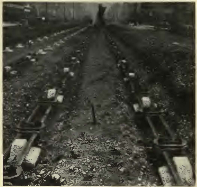
After the trench is graded, precast concrete pedestals are placed in position. The steel framework, made up in 20-ft. sections with anchorages attached, is then placed in position over the pedestals
