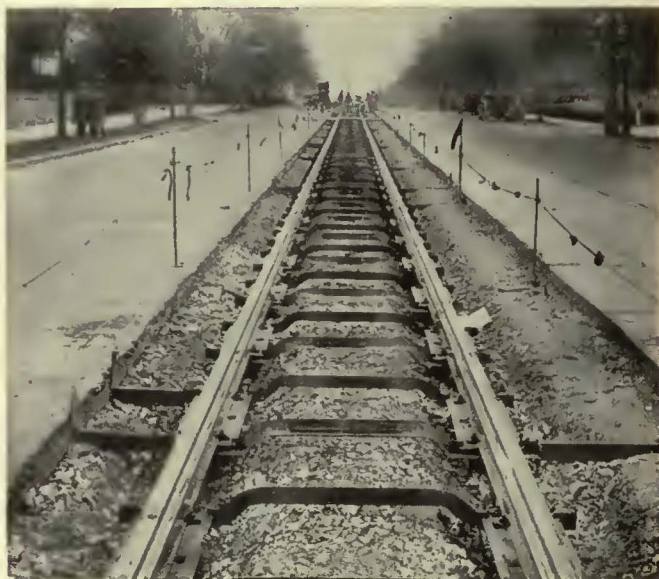
This type of track structure installed by the Capital Traction Company on Connecticut Avenue has now been adopted as standard
