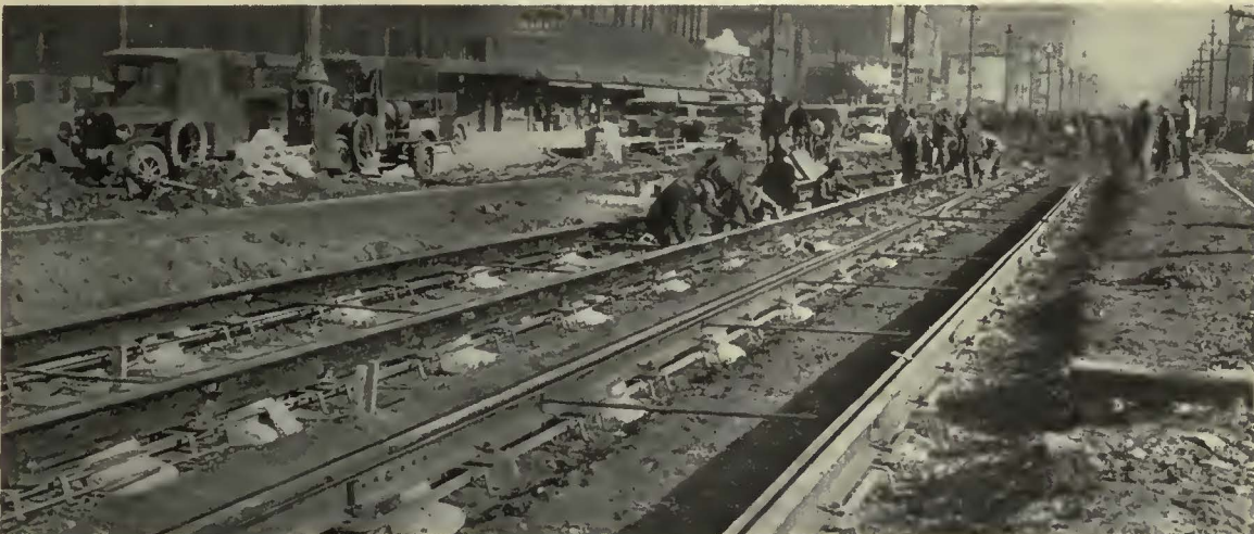
Rails in position with the anchorages attached and clips tightened. Wooden wedge blocks are used on top of pedestals to obtain surface grade adjustment
