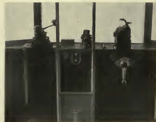
Safety features and simplicity of control permitted the inauguration of one-man operation
