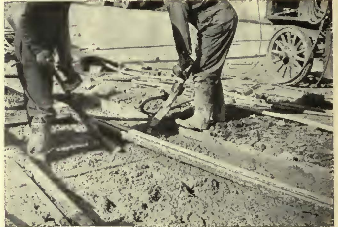
Pneumatic hammers with block tool points were used to drive the concrete thoroughly to place in the foundation
