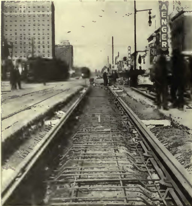
Completed section of tieless track laid in New Orleans. Steel reinforcement is in place and ready for pouring of concrete
