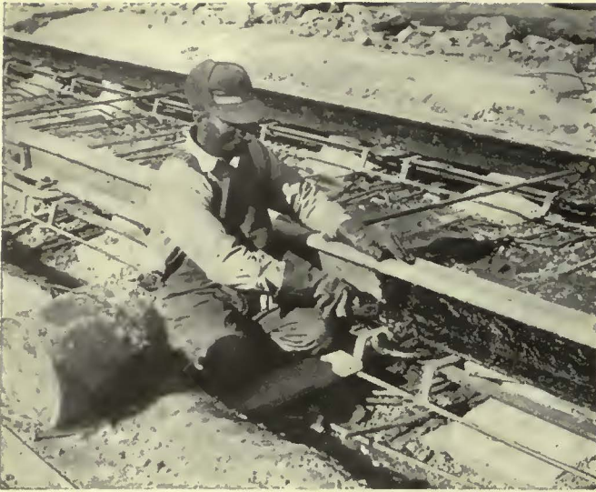
The rail is coated with about \frac{1}{4} in. of plastic asphalt material applied with a paddle as shown
