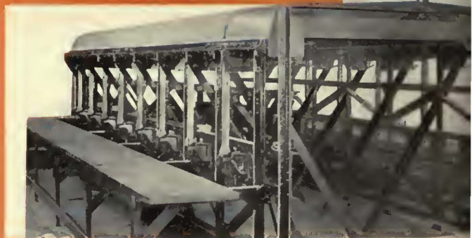
Assembling the roof side posts in a special erection jig. The posts will join the side section at the belt
