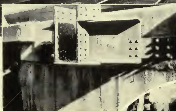
The space for installing supporting bridges is so restricted that in some places they had to be placed on the outside of the retaining wall
