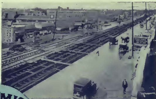
Job on Grand River Avenue, Detroit, completed with standard steel tie and Thermit welded joint construction.
