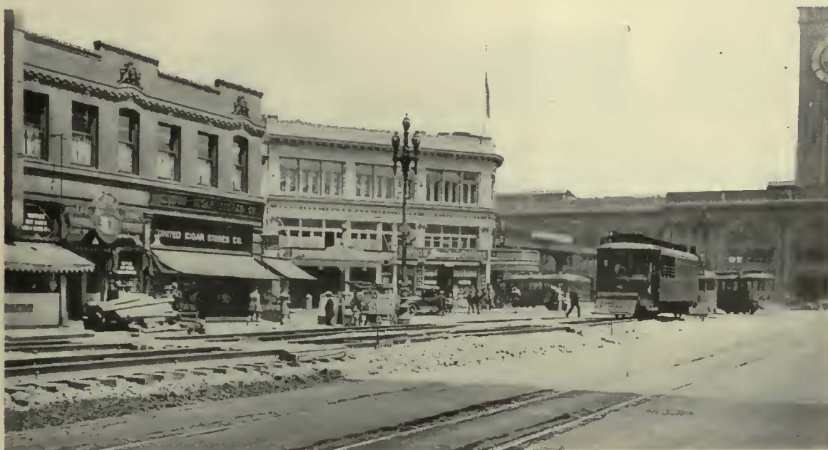
Again in 1923, complete reconstruction of track structure had to be made on Market Street, San Francisco, when street was brought back to official grade
