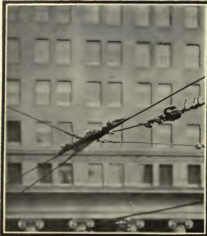
A typical installation of the O-B Duplex Frog in a large midwestern city. Service results are highly satisfactory. Observe the use of the O-B Span Grip Clamp in this installation.
