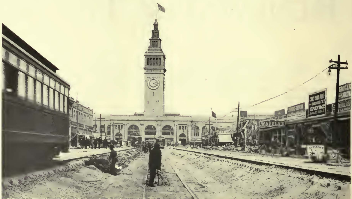
In 1907, track on Market Street in San Francisco had to be raised 4 ft. to bring it back to original grade
