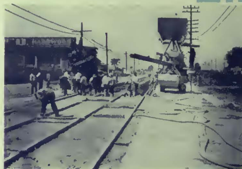
Same job, showing method of concreting using two mixers simultaneously on opposite sides.
