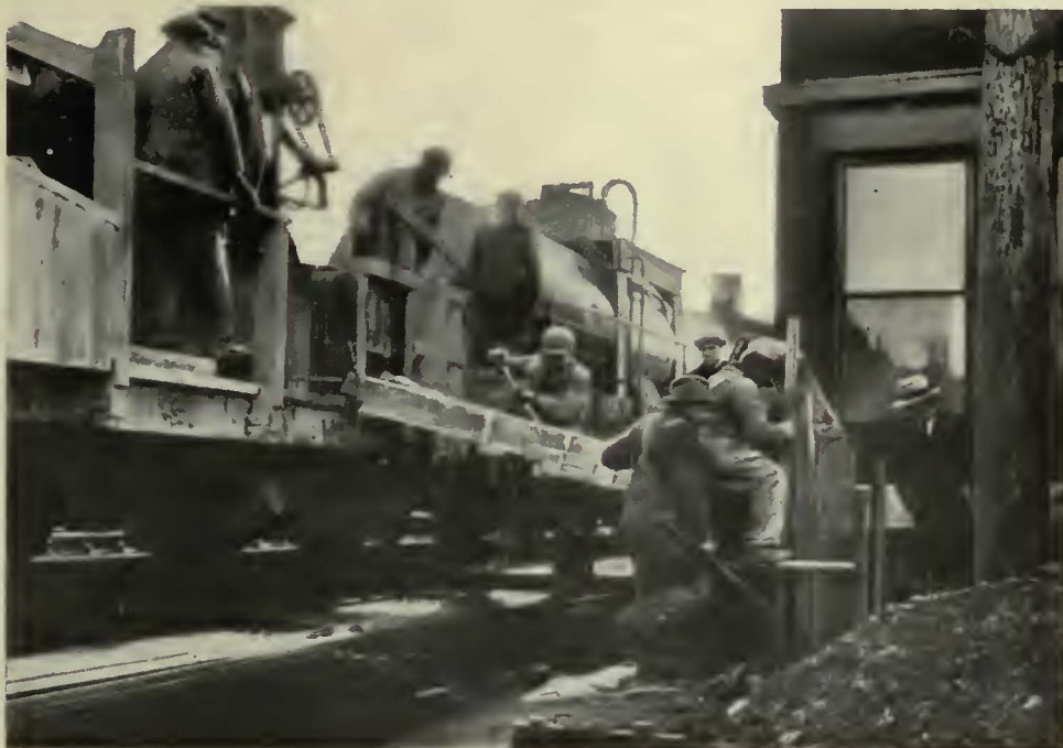
Pouring concrete for a signal bridge foundation under difficulties. By the use of a concrete train no space for installing mixing machinery was needed
