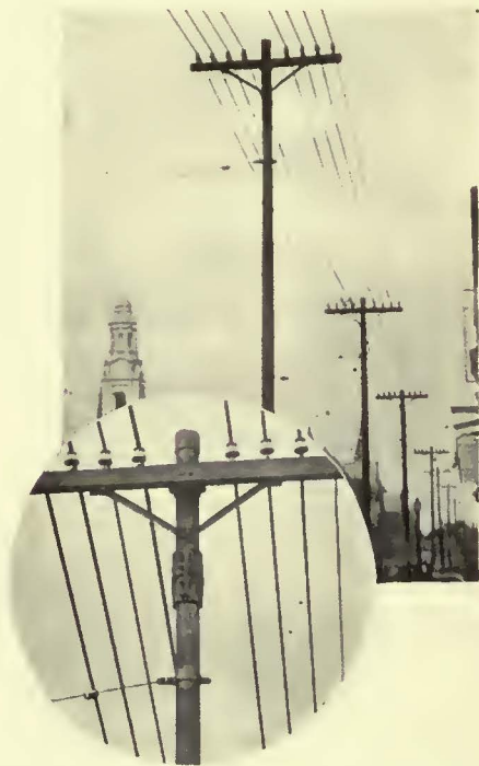
Pole height increased by clamping short extension to top of existing pole
