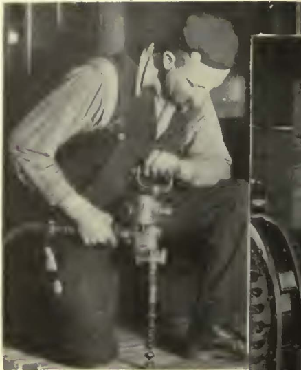
Drilling holes through 2-in. planks at the rate of two a minute.
