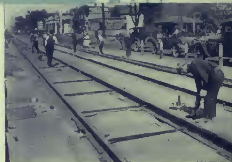
Jefferson Ave. job after new track had been slid into place over night.
