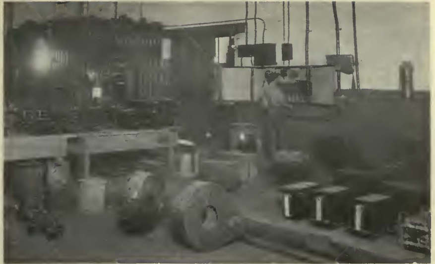
Section of the electrical equipment department where line breakers, circuit breakers, lightning arresters and other apparatus are overhauled
