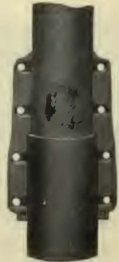
"B" Clamp Reinforcing Corroded Swaged Joint
