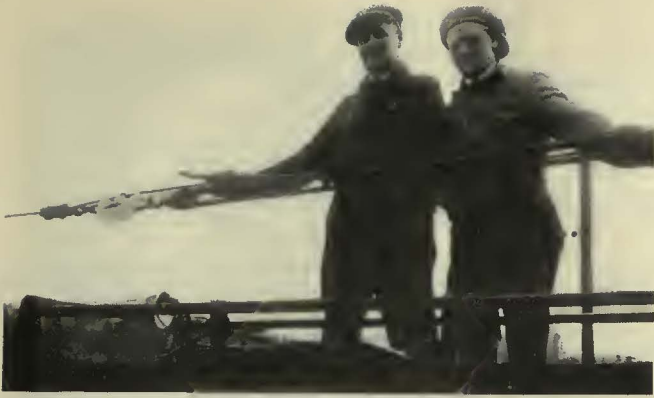
Measuring the trolley wire tension with a dynamometer
