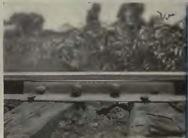
This, and other pictures here, taken on double track. Note conformity of shim to unequal wear in leaving and receiving end of joint.
