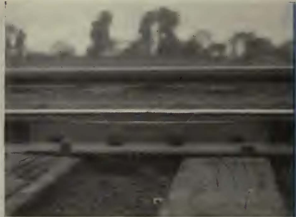
Stark Electric Joint Shim installation. Note conformity to worn fishing angle and restoration of rail to original true surface.
