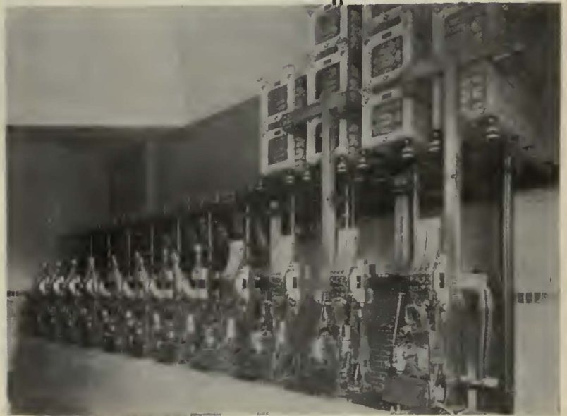
Typical installation of the pedestal-mounted interrupters and load-shifting resistance.
