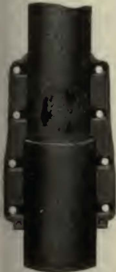
"B" Clamp Reinforcing Corroded Swaged Joint
