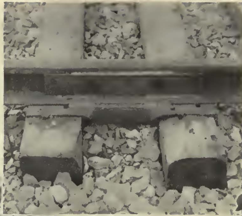
Typical electric seam welded rail joint
