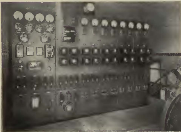
Automatic switching equipment for a 2000-kw. synchronous converter.
