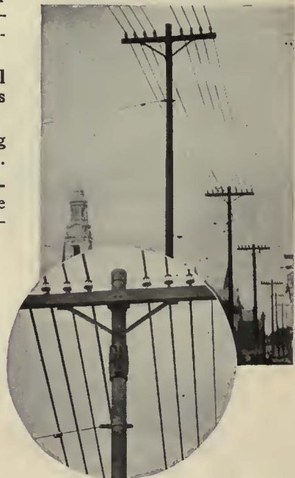
"C" Clamp Supporting Pole Top Extension
