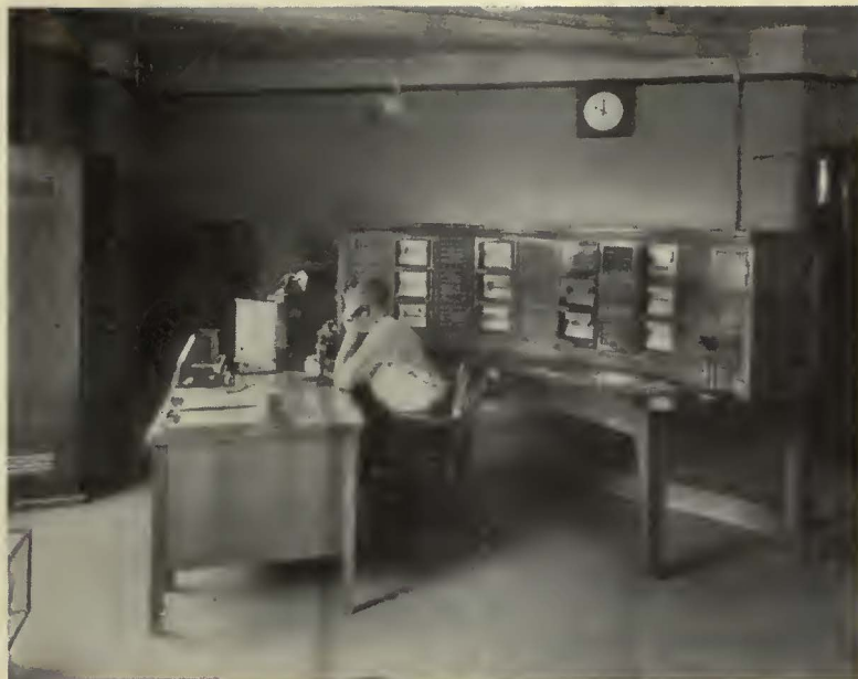
Remote and supervisory control, utilizing various colored lamps for indicated condition of conversion and distribution system control equipment
