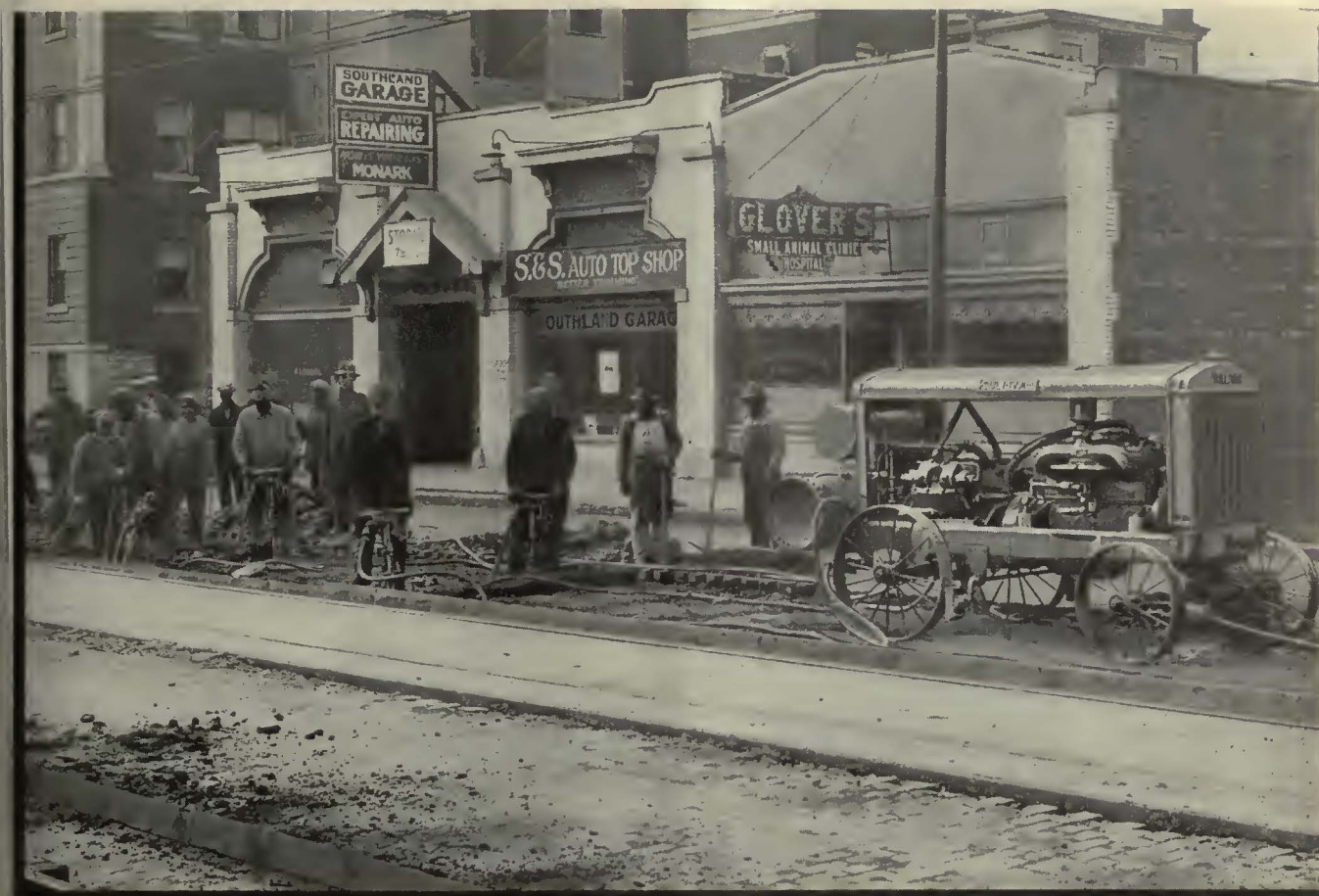
Sullivan 220-ft. Compressor and Sullivan Busters removed 300 ft. of 10-in. Concrete, in 10 Hours.
