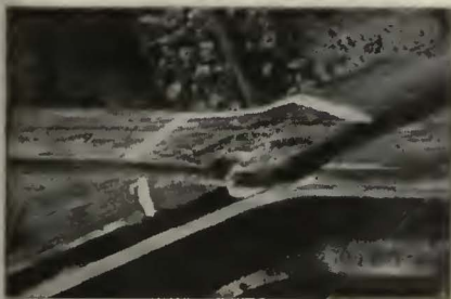
When this crossing on a main line failed it was quickly welded with TIMANG and kept in service on this line for four months, and then removed to another piece of track.
