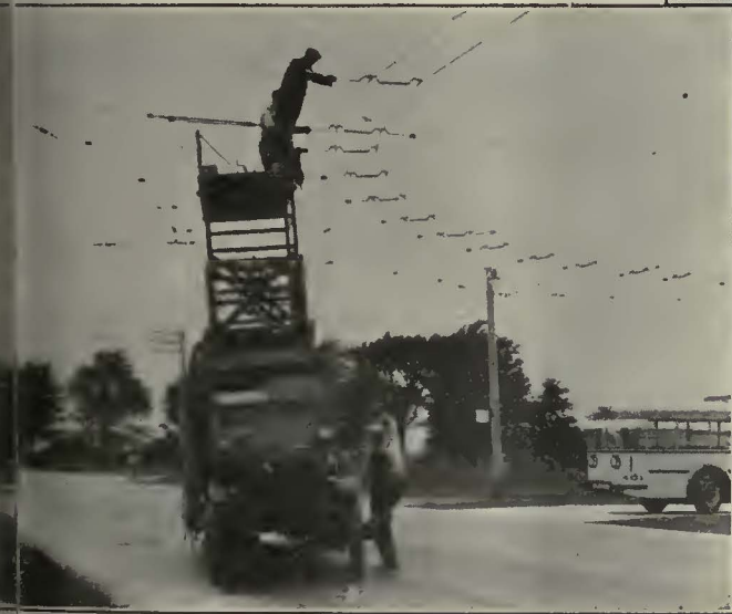
(Right) Crew working on loop at River Rouge Park terminals of the Plymouth Road Trolley Bus line. O-B Single and Double curve hangers, with special wood strain insulators are used.
