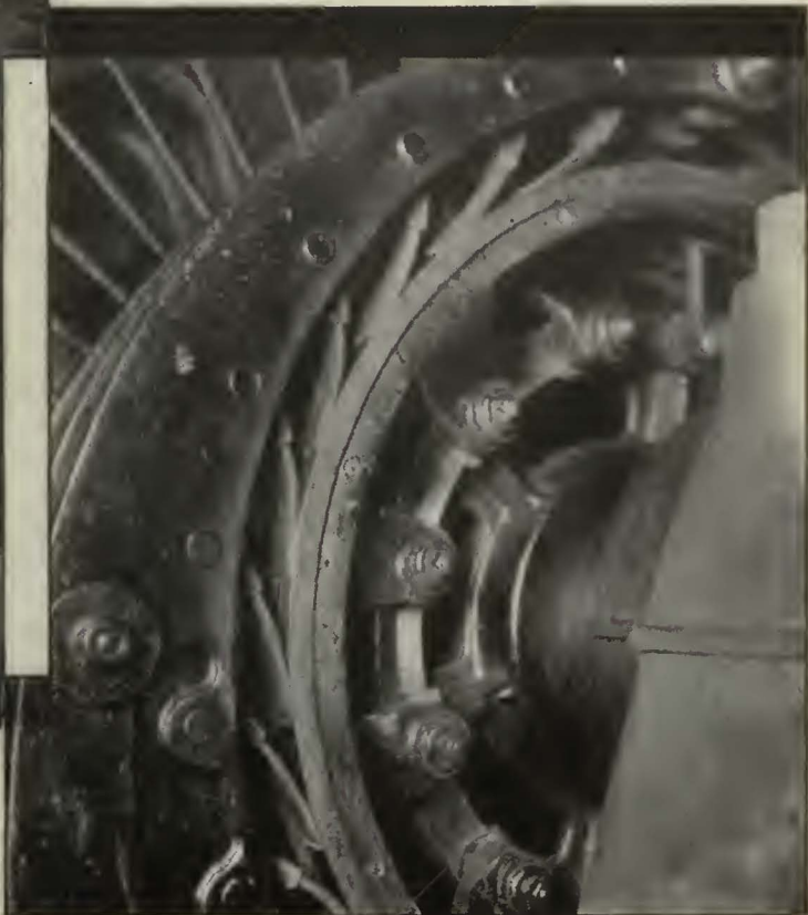
Slip-rings of rotary converter equipped with old-style copper-leaf brushes
