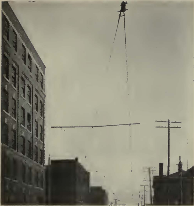
Temporary crossover used by the Cleveland Railway is easily and cheaply installed
