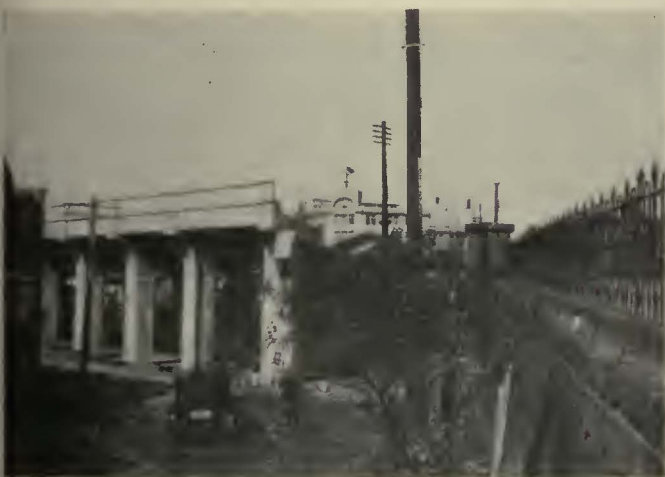
A Difficult Piece of Diversion Work on the Elevated Electric Railway, Now Under Construction in Kobe, Japan
