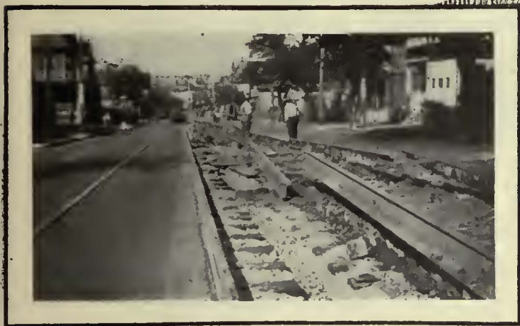
Providence carried traffic through on one track while the other was being reconstructed.
