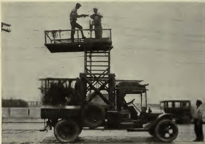
Public Service line crew renewing trolley ears. Periodic renewal has prolonged life of trolley wire approximately 50 per cent
