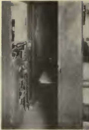
Control equipment is grouped in a permanent cab at each end of the car
