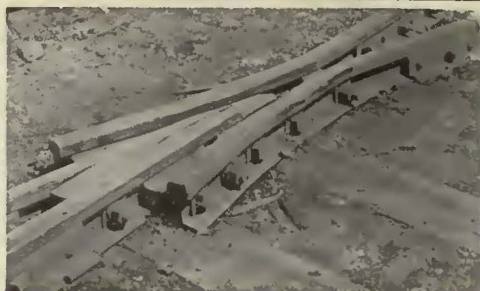
Plain bolted frog which had been worn out, and quickly reclaimed by welding with TIMANG.
