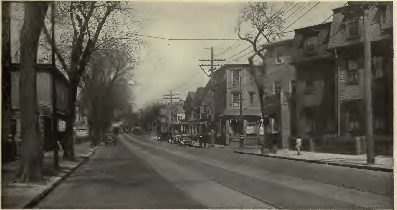
Track in Somerville, Mass., restored to good condition after 30 years of service
